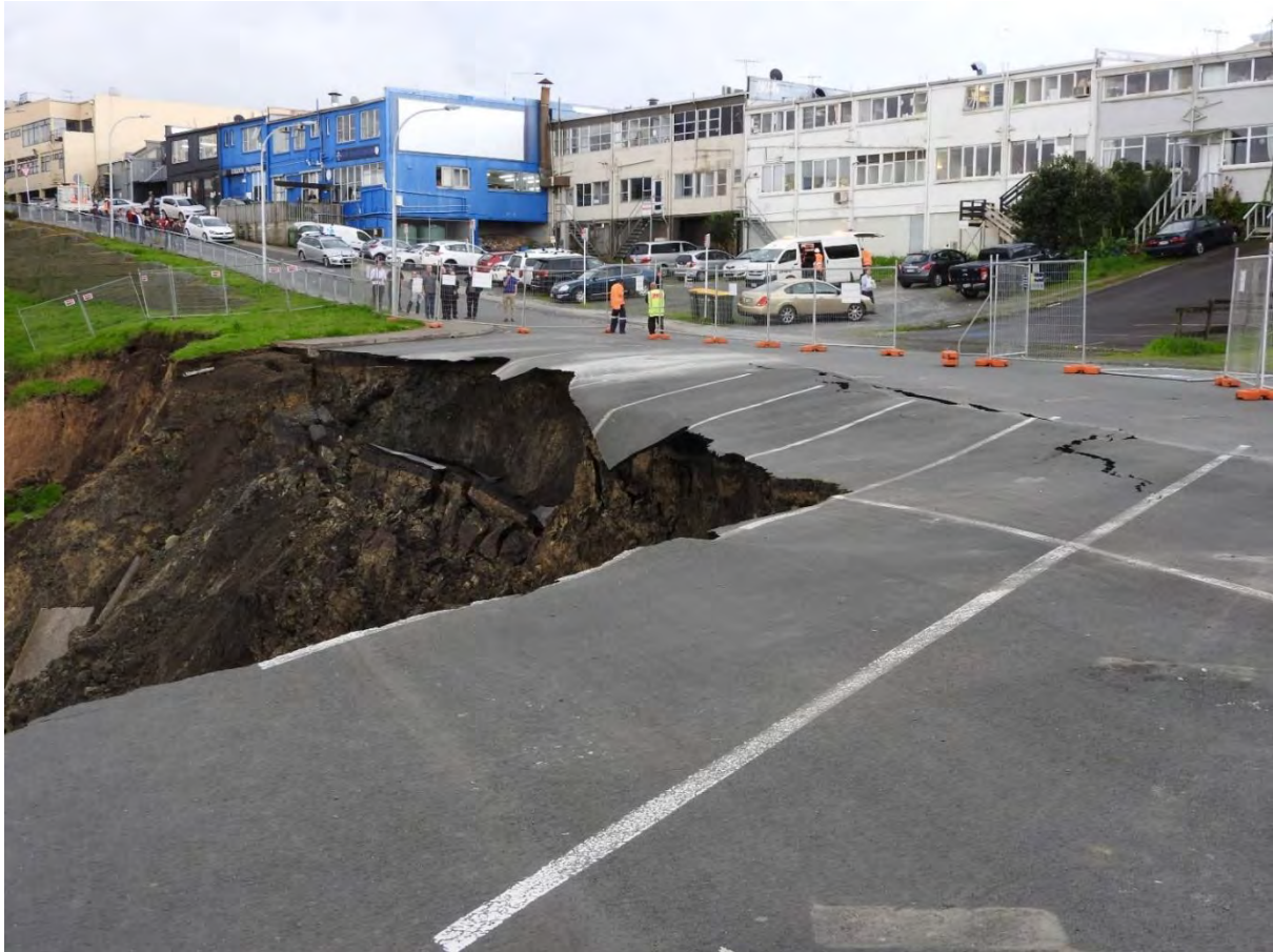
Figure 10: The Rawene Road landslide in Birkenhead, following a storm in 2017 (Source: Auckland Council)
