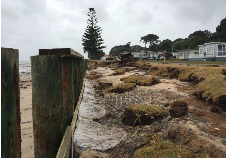
Figure 32: Damage caused by a storm event in early 2018 at Hudson Beach along Awhitu Peninsula (Source: Auckland Council)
