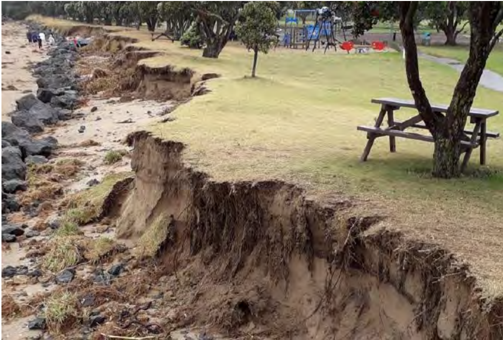
Figure 9: Coastal erosion at Stanmore Bay, Whangaparāoa following January 2018 storm events. The event lowered beach levels, exposing legacy buried rock and eroding the reserve edge (Source: Auckland Council)
