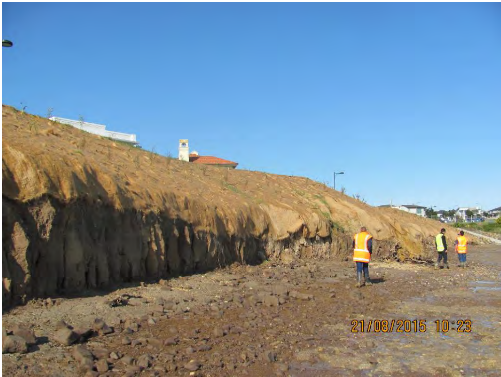
Figure 45: Council works to mitigate erosion of esplanade reserve and footpath in 2015 (Source: Auckland Council)
