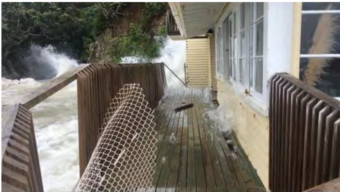
Figure 13: Storm damage to Rakino Community Hall (Source: Auckland Council)
