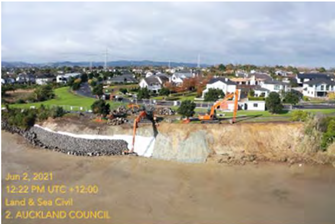
Figure 46: Karaka Harbourside - Stage two rock revetment, completed in 2021 (Source: Land & Sea Civil Ltd)
