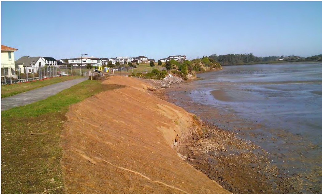
Figure 42: Karaka Harbourside esplanade reserve following removal of undermined tree stumps and re-grading of cliff edge in 2015 (Source: Auckland Council)
