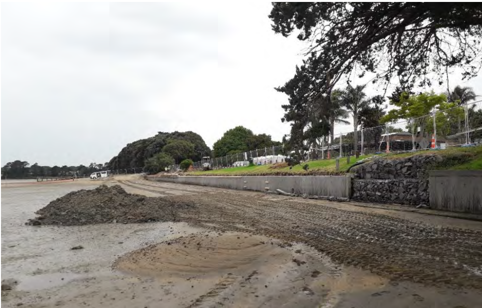
Figure 36: Repairing of an existing failing seawall along the western end of Sandspit Beach. (Source: Auckland Council)
