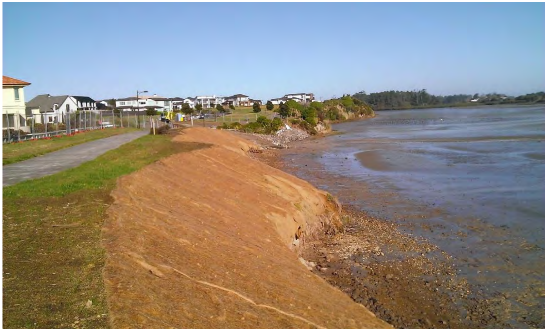
Figure 22: Karaka Harbourside esplanade reserve following removal of undermined tree stumps and re-grading of cliff edge in 2015 (Source: Auckland Council)
