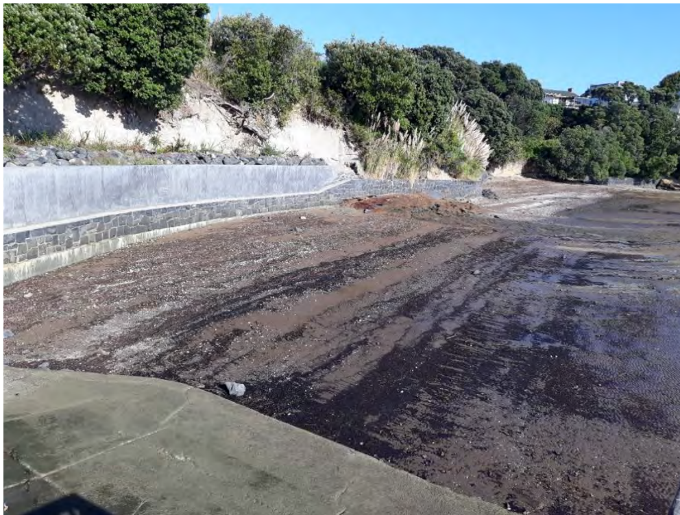
Figure 37: Mass concrete retaining wall (Auckland Council asset) constructed at Andersons Bay, Glendowie (Source: Auckland Council)
