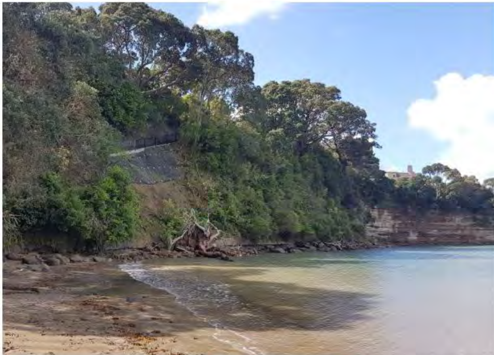
Figure 8: A typical Auckland East Coast cliff showing a recent repair to reinstate a footpath damaged by cliff instability (Source: Roberts, R., N Carpenter and P Klinac. (2020). Predicting Auckland’s exposure to coastal instability and erosion (Auckland Council technical report, TR2020/021), Auckland Council, pg. 6)
