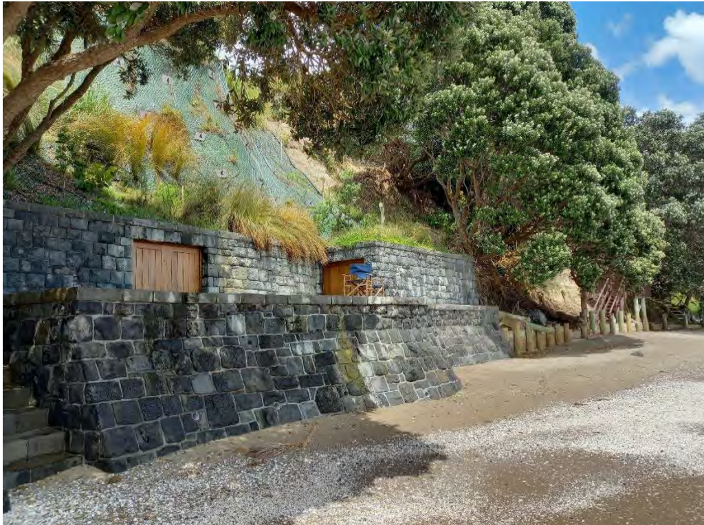
Figure 38: An example of soil nails and hard coastal protection structure at Beachlands (Source: Auckland Council)
