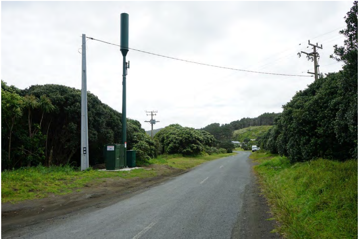
Figure 39 A new cell tower near Bethells Road near Bethells Beach (Kensington, 2023).
