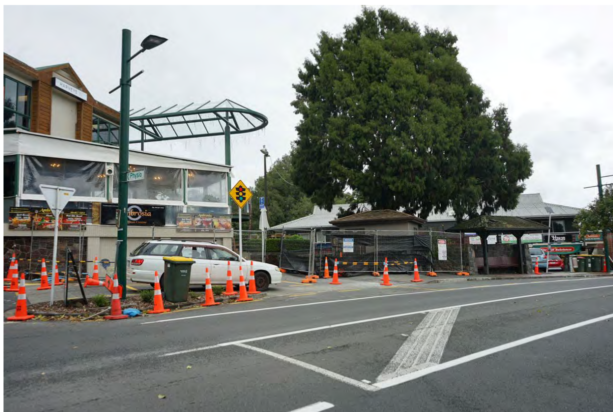
Figure 8 New public toilet block in Titirangi township under construction in late 2022 (Kensington, 2023).
