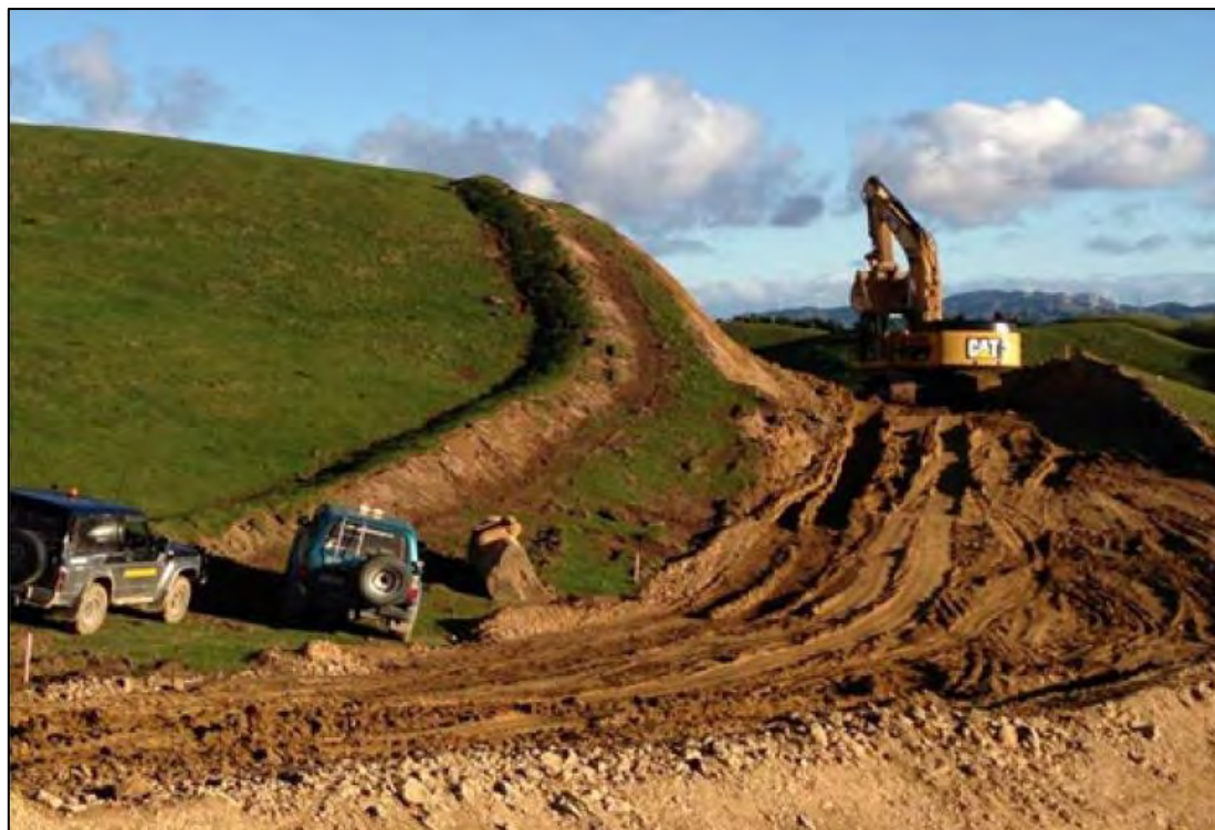
Figure 8: Photograph of Clean Water Diversion Bund
