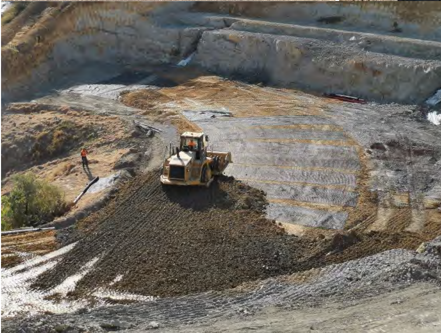
Inset 7: Construction Photos for Compliance stage (shear key, benching out, drainage). Butress filling will be placed upon the prepared ground and final design levels achieved to enable urbanisation.
