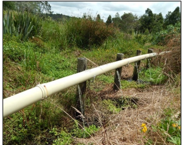
Figure 2-16: Beachlands WWTP Overland Flow Distribution Pipe
