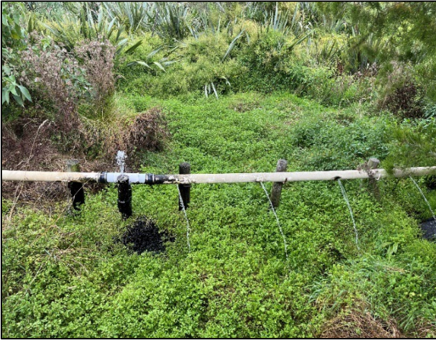
Figure 2-15: Beachlands WWTP Overland Flow Distribution Pipe
