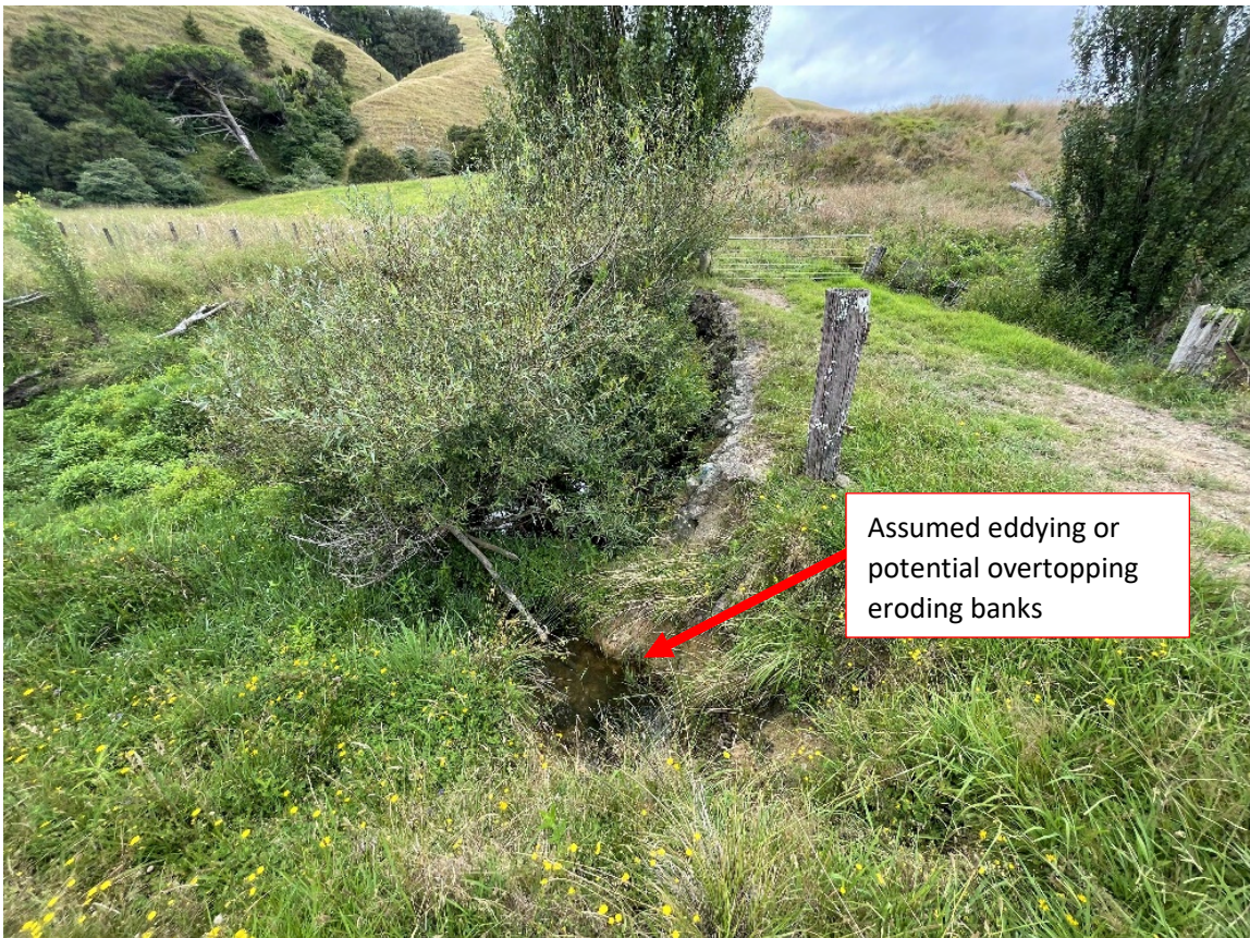
Figure L: Erosion Downstream of DN 1200 Farm Culvert (18/01/2024)
