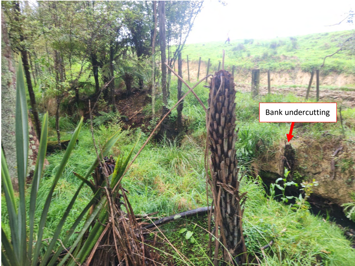
Figure E: Undercutting of Stream Bank Example 2 (06/09/2023 – Facing Upstream)
