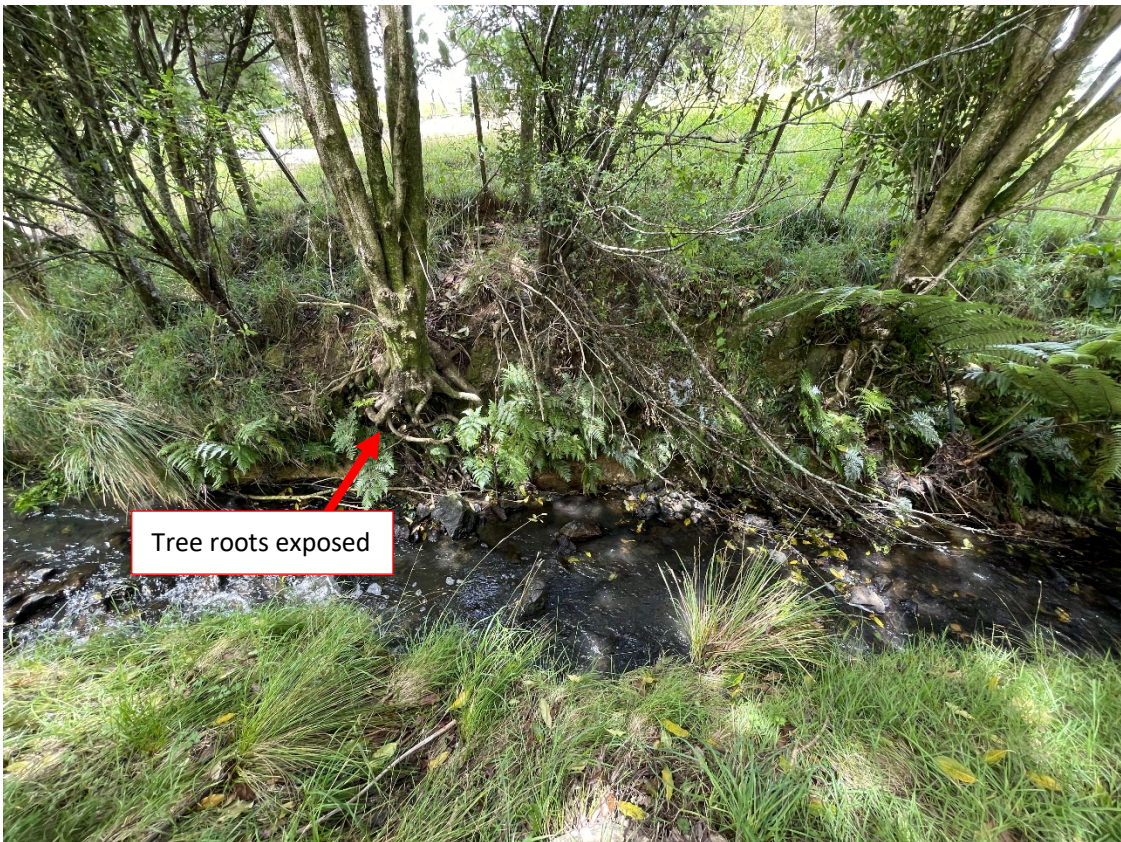
Figure J: Bank undercutting downstream of Bridge (18/01/2024)
