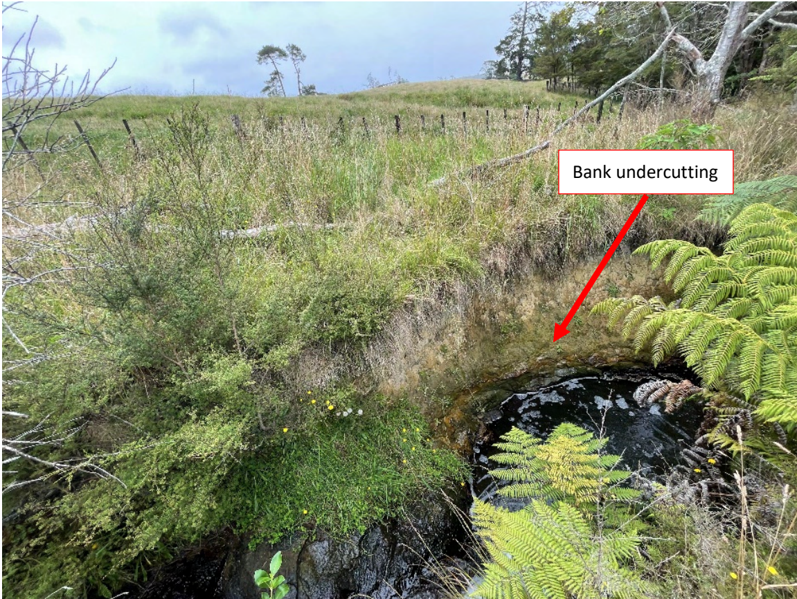
Figure C: Undercutting of Stream Bank (18/01/2024 – Facing Downstream)
