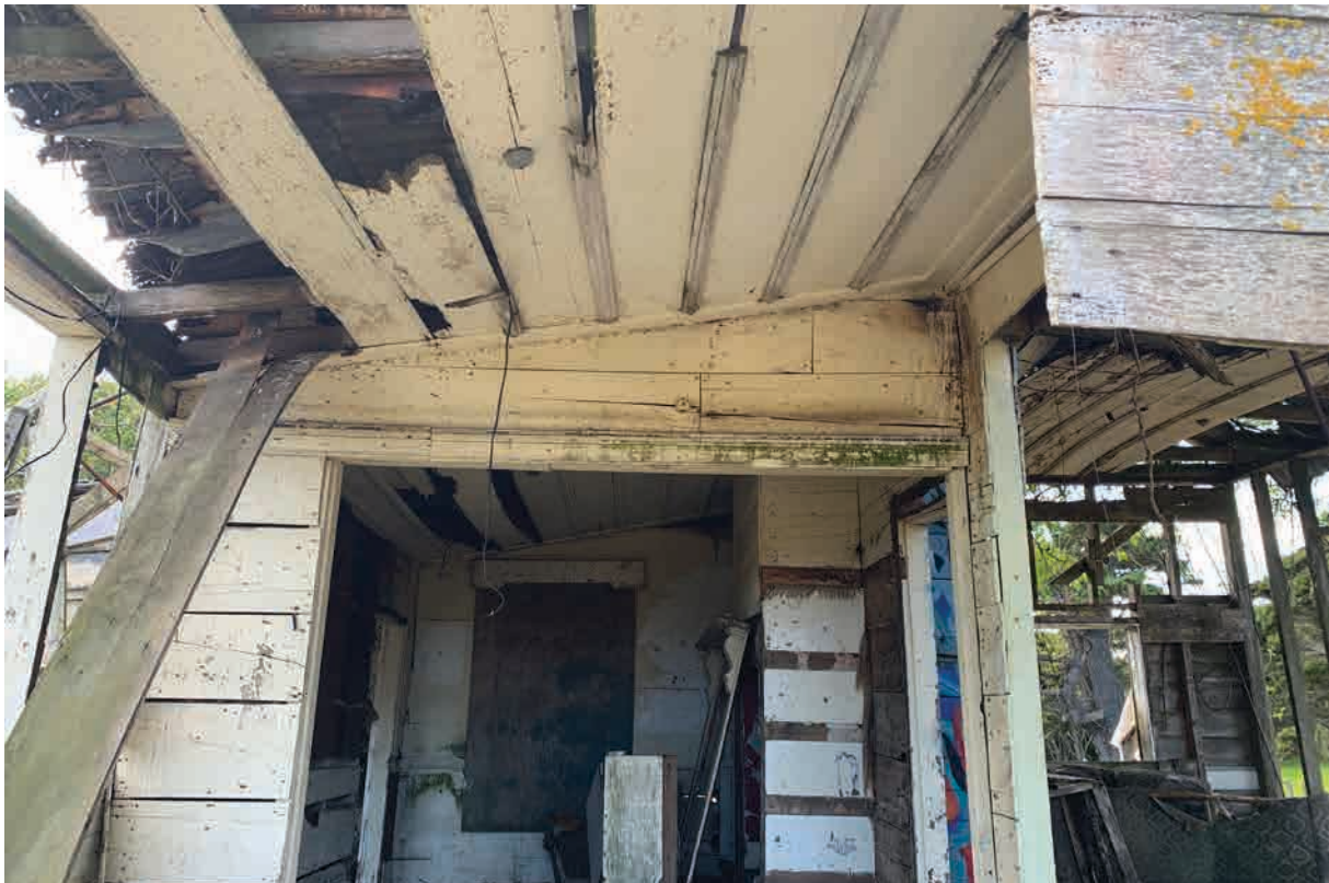
Figure 19. Horizontal sarking and board and batten ceiling in the dilapidated cottage Q11/614.
