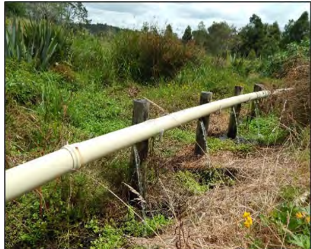
Figure 2-16: Beachlands WWTP Overland Flow Distribution Pipe
