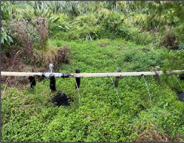
Figure 2-15: Beachlands WWTP Overland Flow Distribution Pipe
