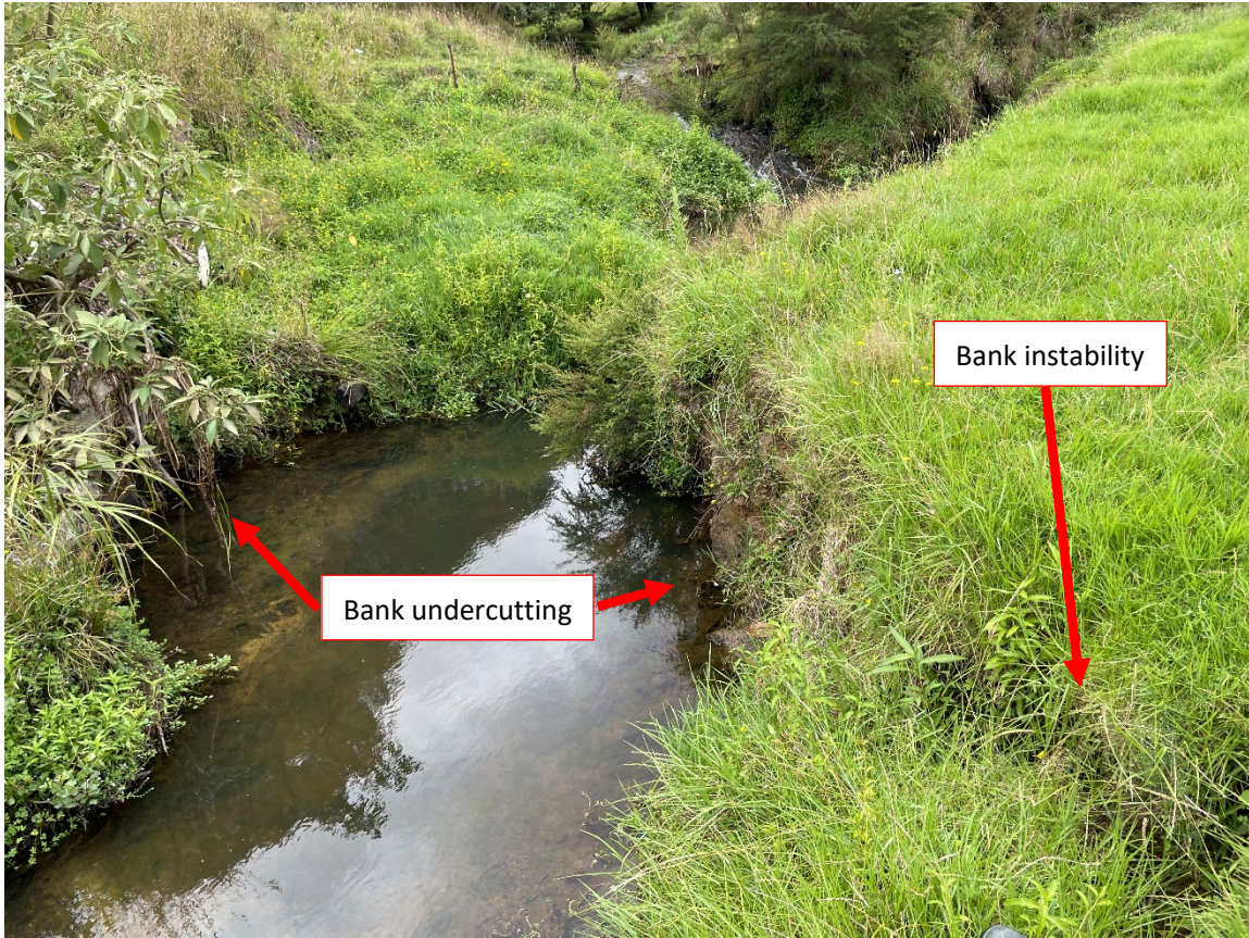
Figure O: Bank undercutting at Point C (18/01/2024 - Facing Upstream)
