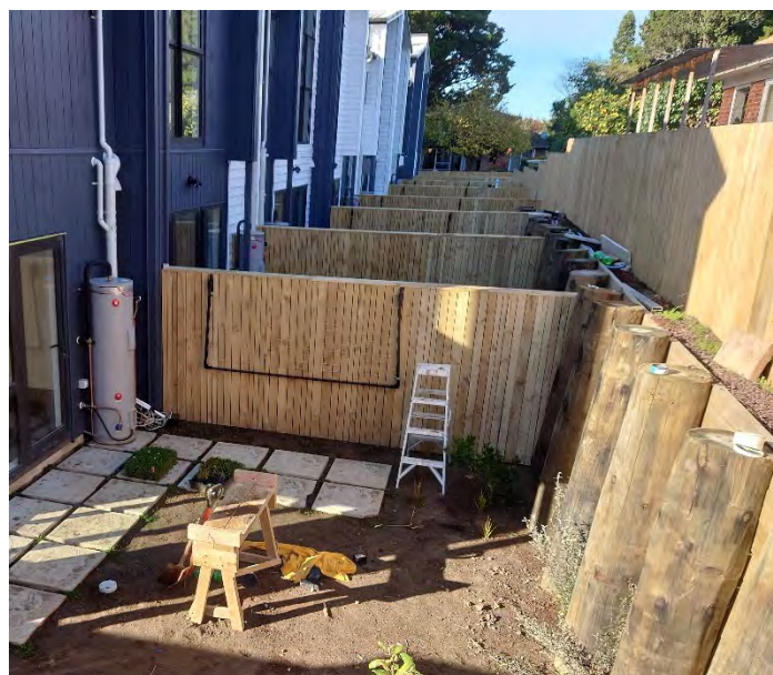
Figure 3: This photo shows a high retaining wall combined with a fence can cause both shading and dominance effects on the amenity of the outdoor living space. However, privacy and dominance effects of the new development on the adjoining site are reduced with the change in level created by the earthworks. This shows there can be positive and negative outcomes from earthworks.
