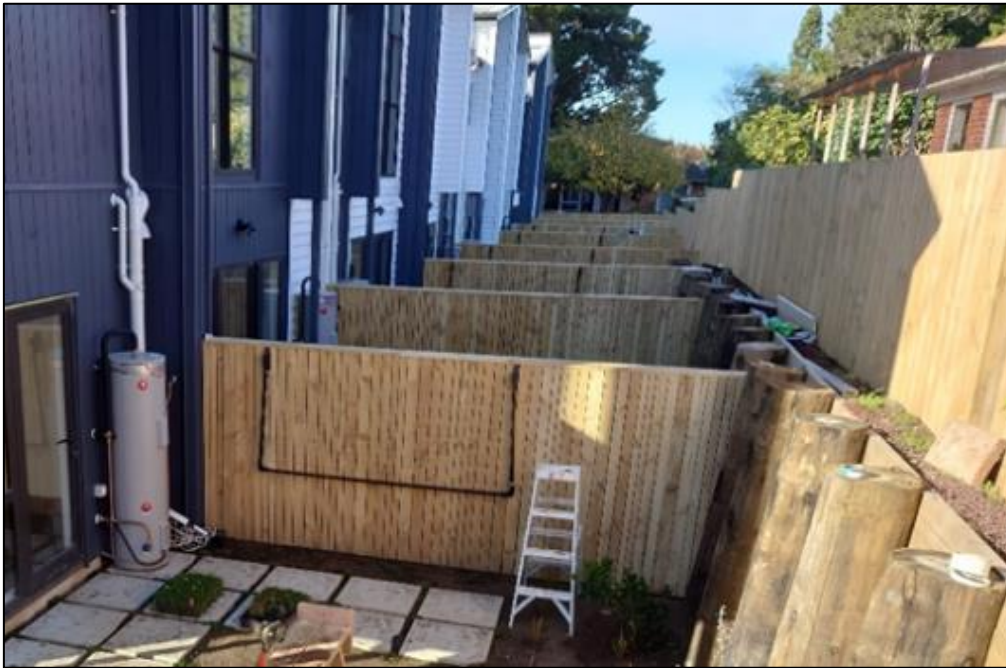
Figure 30: Photograph of effects of fencing on outdoor living areas when built upon retaining walls.
