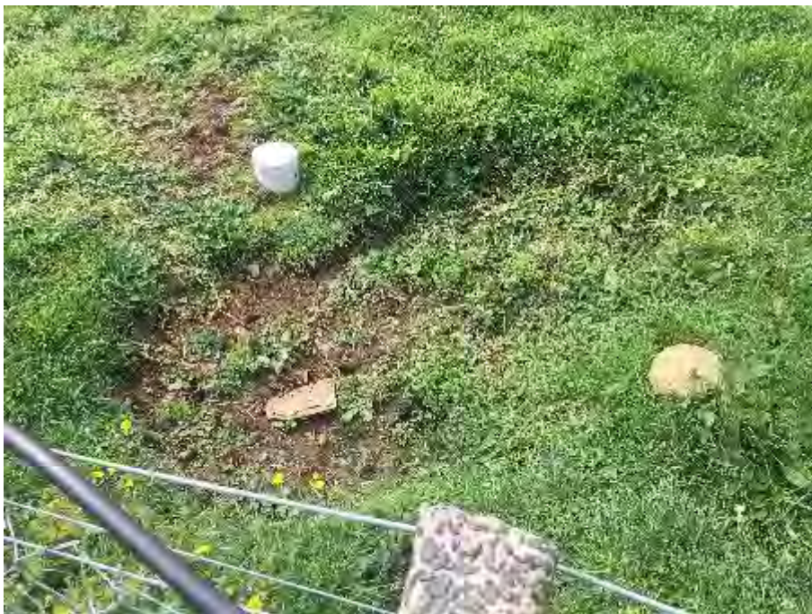
PLATE 4: BREATHER VALVE FOR SEPTIC TANK ASSOCIATED WITH THE ORIGINAL DWELLING
