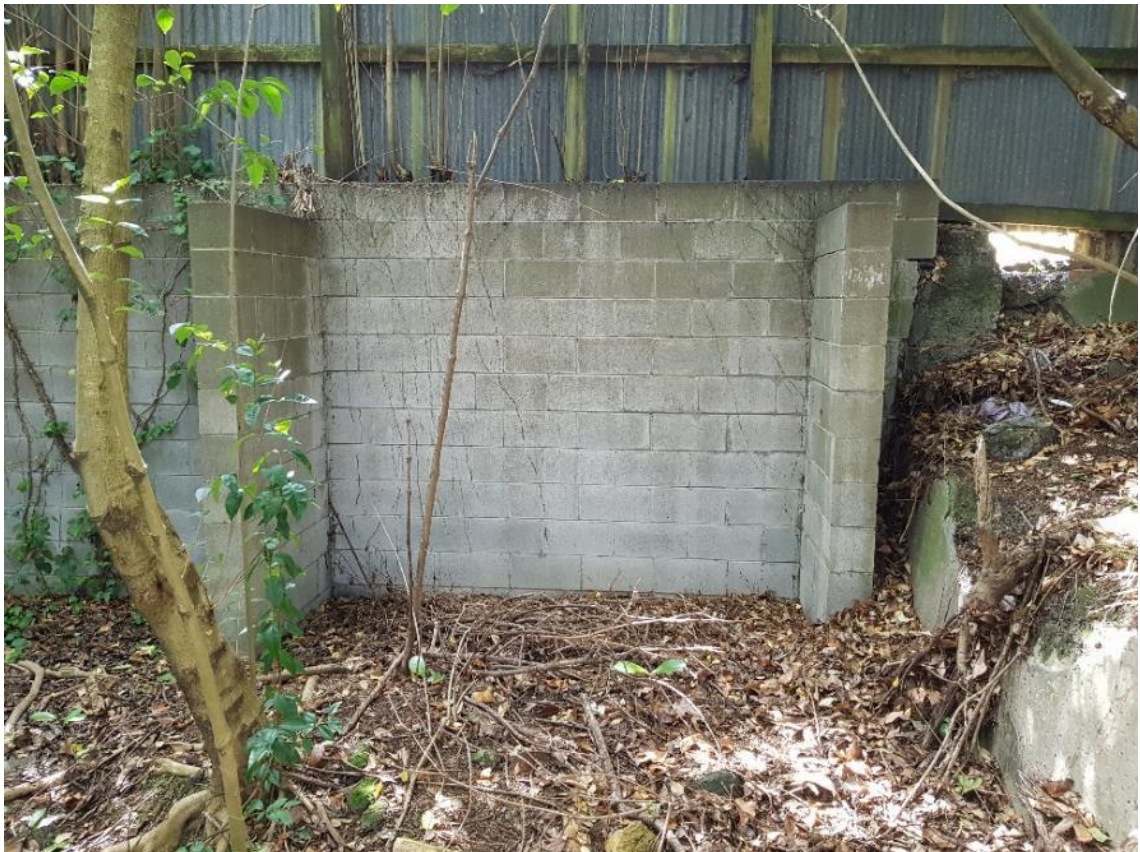
Figure 23. A retaining wall of concrete blocks adjacent to the feature is on the Ladies Mile boundary
