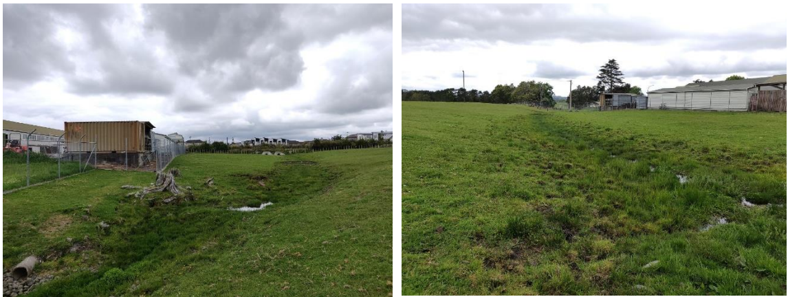
Figure 17. Continuation of stream in southeastern corner of 102-102A Totara Road, looking south along eastern property boundary showing concrete culverts (left photo); and facing north/northeast with eastern property boundary on right (right photo)
