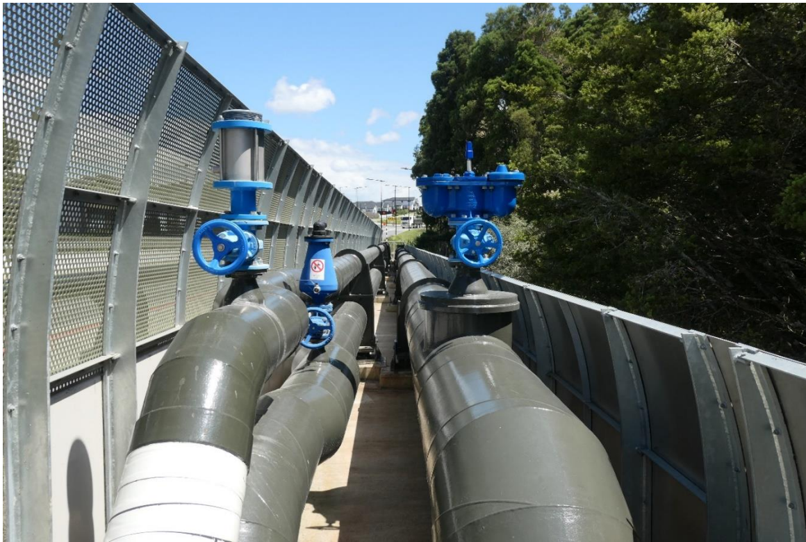
Water and wastewater pipes on Weiti Bridge, Milldale.
