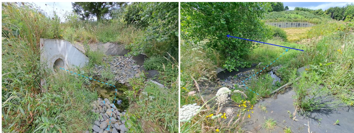
Figure 9. Existing culvert wingwall structure. The light blue dashed line indicated the stormwater flow path (including a 90 degree direction change) into the stream (dark blue line).
