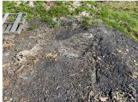
#4 Rubbish burning area on asphalt chip
