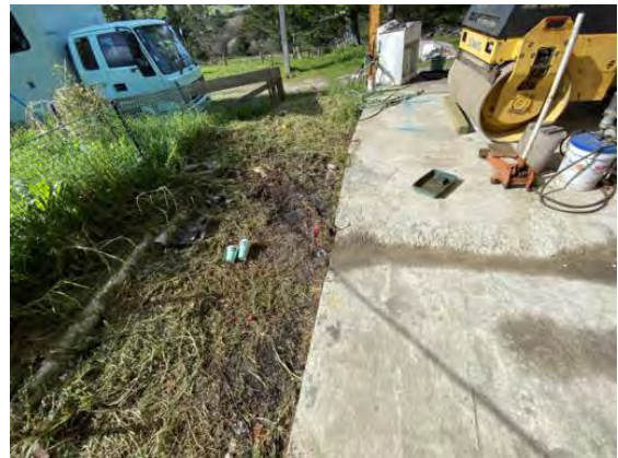
#21 – Container shed oil staining
