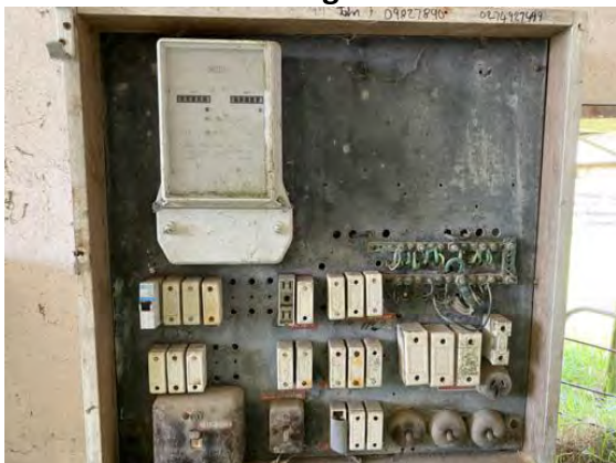
#5 – Milking shed switchboard
