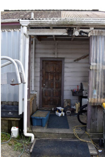
Fig. 63 Non original rear door, currently used as the primary entry into the dwelling,
