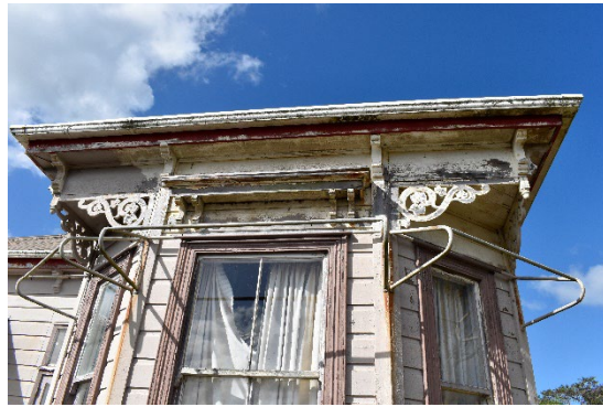
Fig. 62 Timber brackets under the soffit, decorative fretwork, and later intrusive metal frames attached for awnings.
