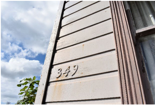
Fig. 61 The former street number on the principal elevation. Note this number is not orientated towards the street.
