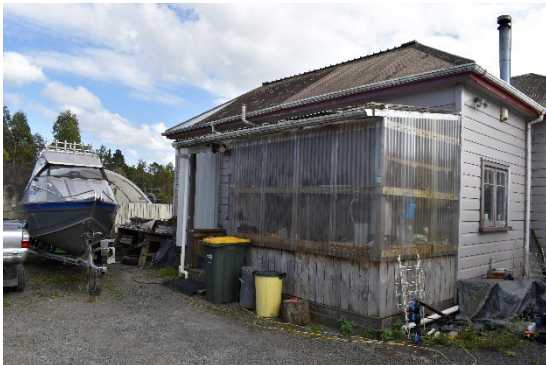
Fig. 59 Looking north towards the rear of the villa and a later lean to addition.
