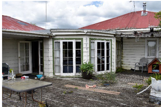
Fig. 40 Looking south toward the radial form connecting the original dwelling (right) to the 1984 addition (left),
