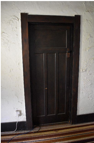
Fig. 50 Doors within the original portion of the dwelling feature doors and architraves typical of the 1920s design style.
