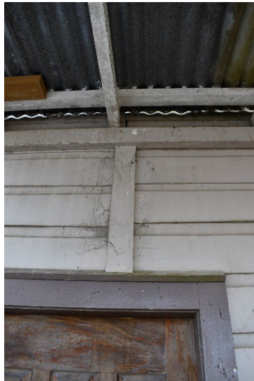
Fig. 64 A join in the weatherboards above the rear door is indicative of where the dwelling was split to allow for its relocation.
