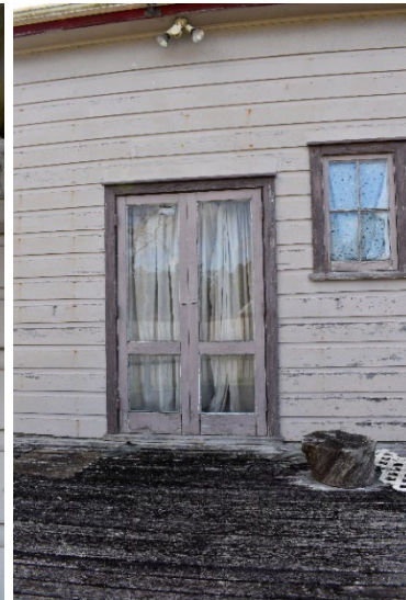
Fig. 65 The western elevation showing non-original outward opening glazed doors and a 4-pane casement window.
