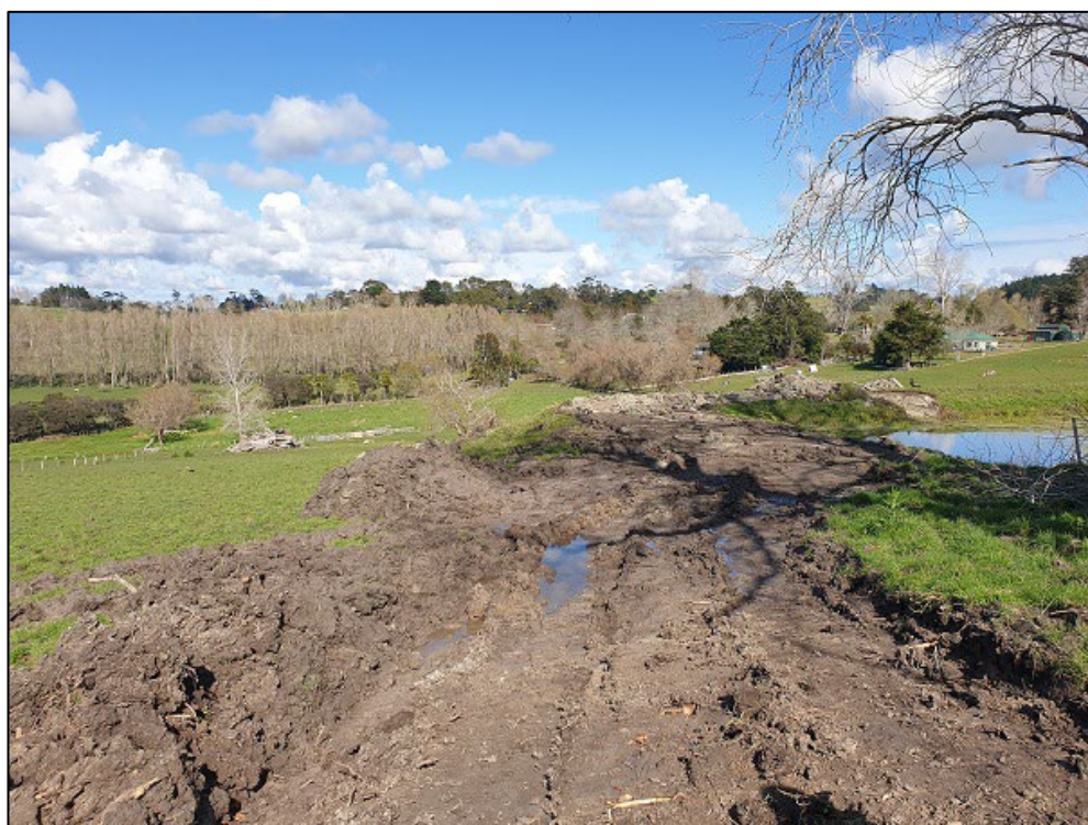
Figure 49. Earthworks at second pond to the west of the possible well location
