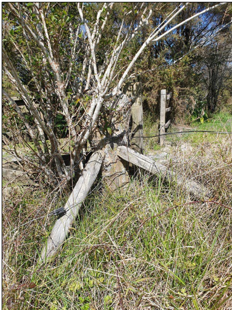
Figure 56. Large corner post the creek crossing with two stays set within it
