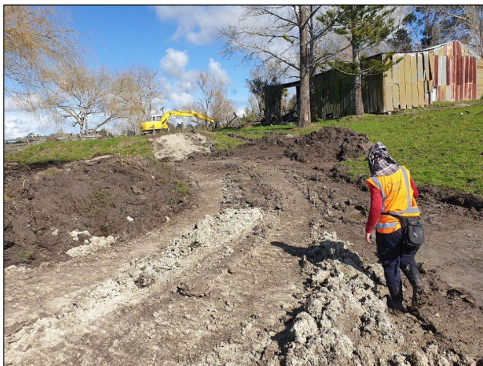
Figure 47. Cut access track to the southeast of the shed shown in Figure 3. Redeposited grey clay visible in foreground and dark topsoil spoil
