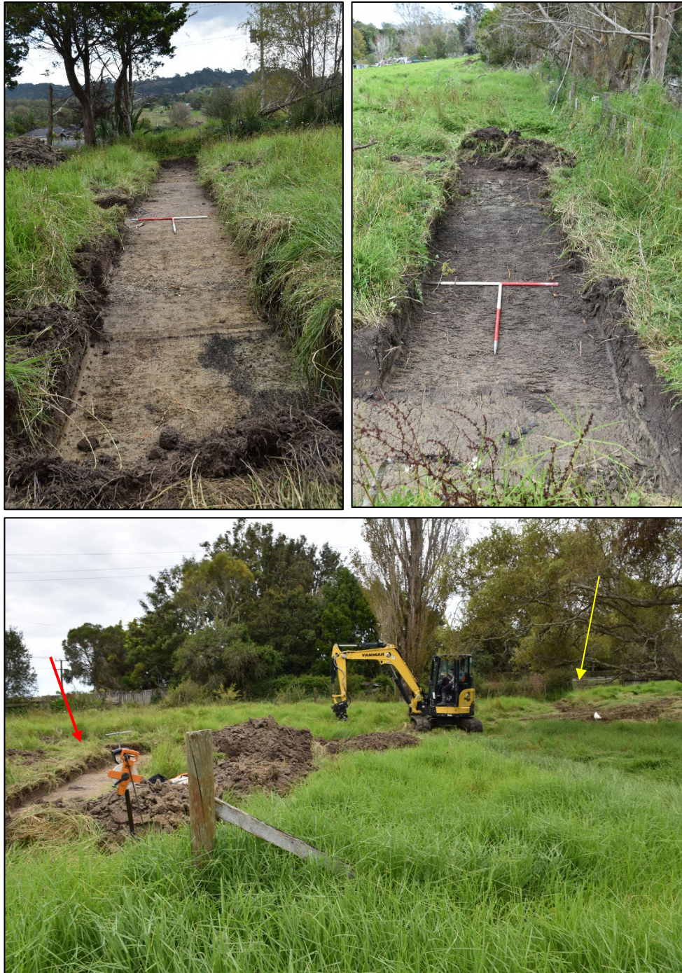
Figure 21 Trench 6 – longest trench on top left, facing north; short trench by road frontage on top right; and Trench 6 with postholes on the left (red arrow) and backfilled Trench 5 on the right (yellow arrow), facing northeast (1m scale bars)
