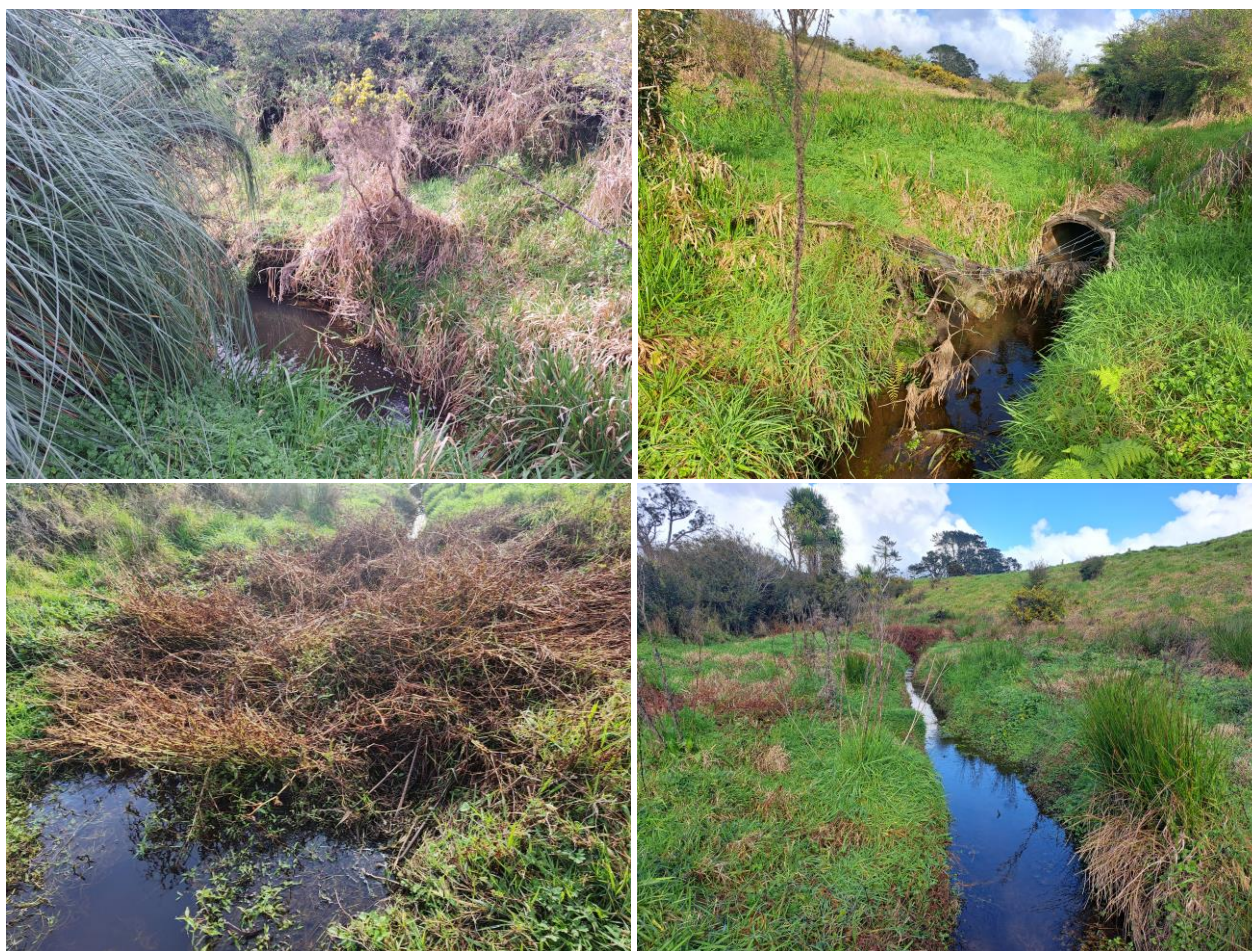
Figure 20: General characteristics of the Trig Stream. Low lying culverts (top right) were identified on site, alongside unidentifiable crossings obscured by vegetation (bottom), with visible shifts in the water level on either side (bottom right).
