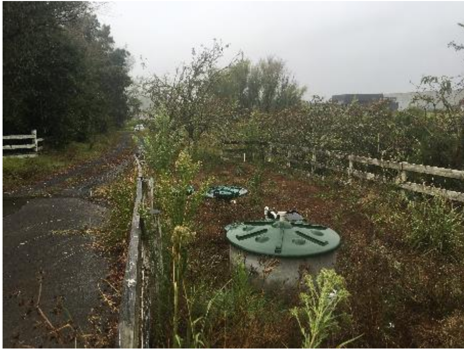
PLATE 9: SEPTIC TANKS ON 100 HOBSONVILLE RD
