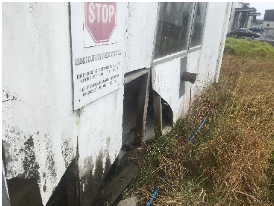
PLATE 2: BROKEN FIBRE CEMENT PANEL ON EASTERN END OF POULTRY SHED
