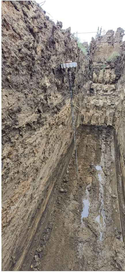
Figure 1 - Test Pit 1 (1.0m Weak Fill)
