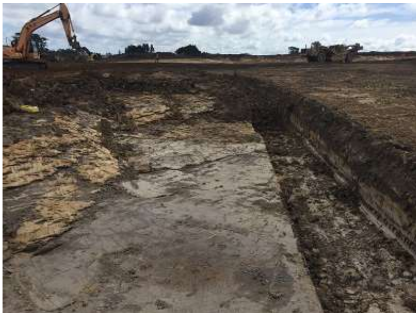
Photo of site showing area where topsoil previously identified under fill has been stripped out (centre). A small wedge left to remove in the side of cut of swale at right.
