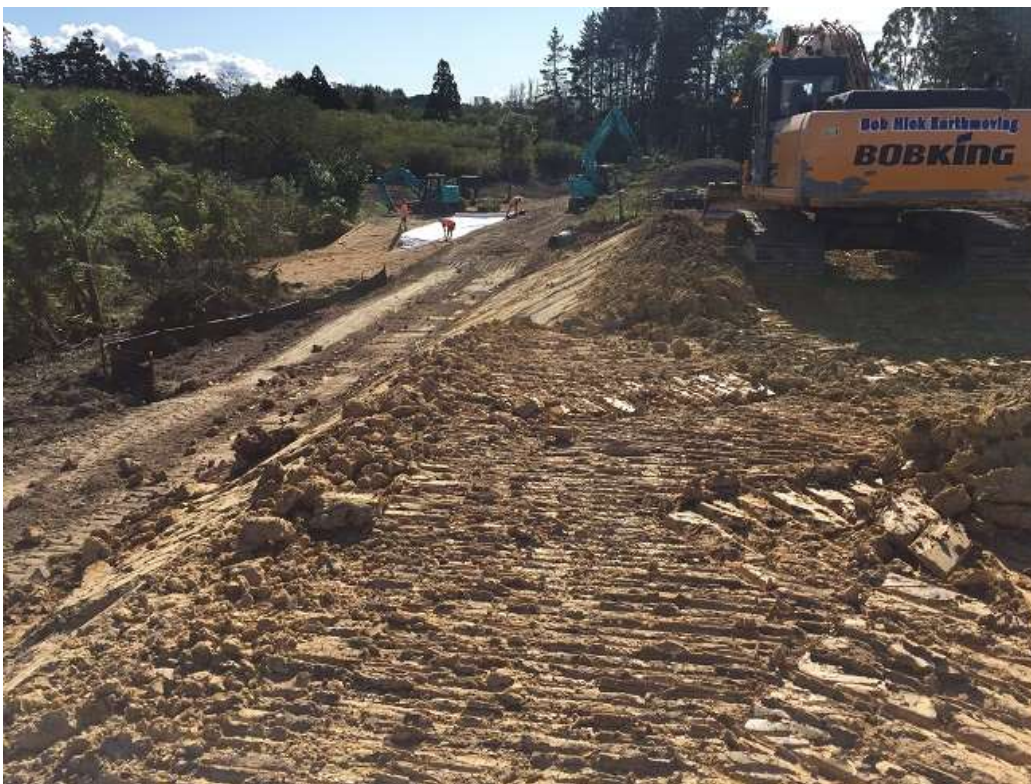
Fill batter being formed in north-western part of site under future Spine Road.
