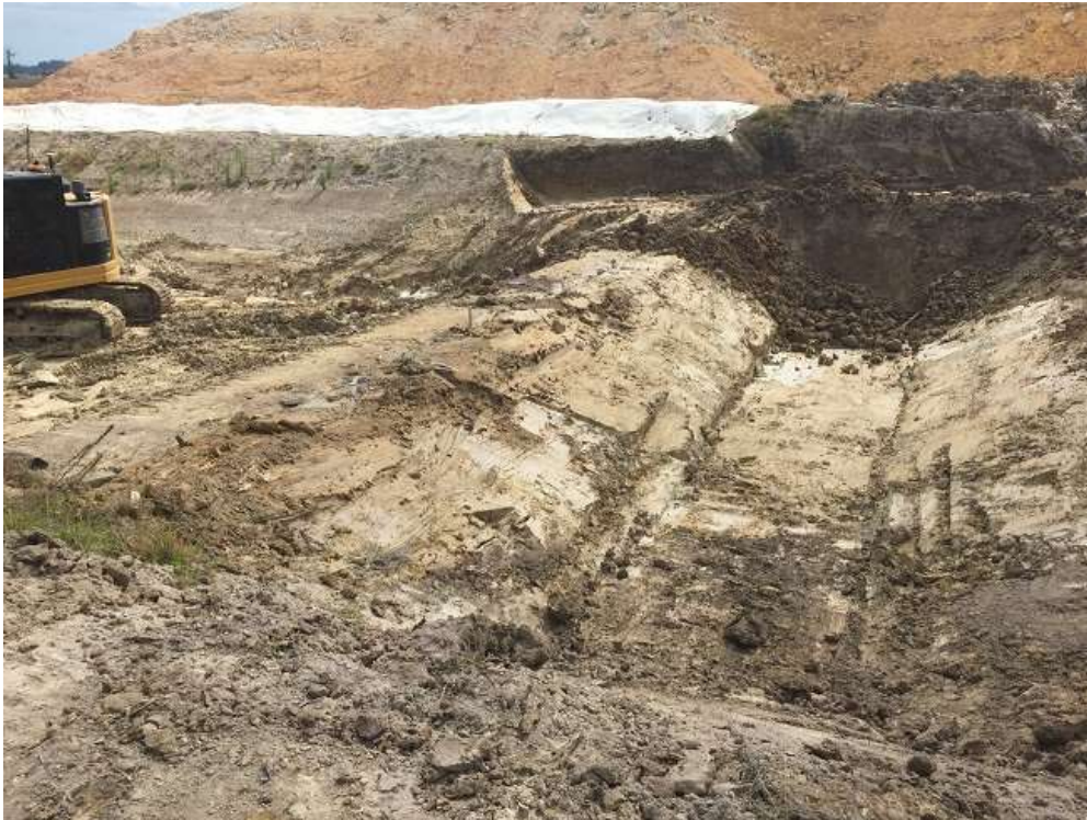
Forebay area stripped - the loose bits tracked in by roller visible at rear were cleaned up while on site.
