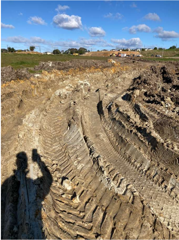
Looking from the old stockpile towards Lot 8 at the significant rutting.
