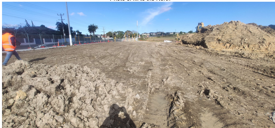
Photo of fill to the South toward cnr Spine & Hobsonville, as well as remaining stockpile to the right.
