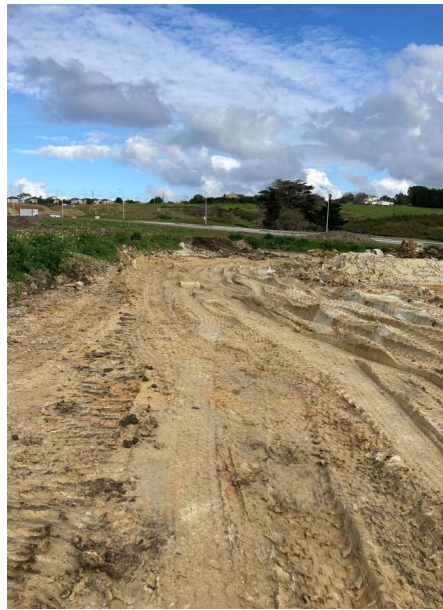
Rutting evident to the south of the Lot 10 stockpile.
