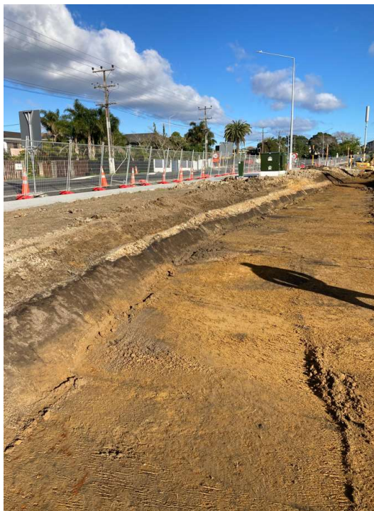
Photo of haul road on Lot 5 looking to the south. Note the topsoil visible in the sidewalls.
