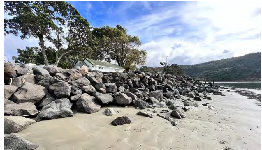
Condition of Seawall before (July 2023): Rock migrated onto the beach.
