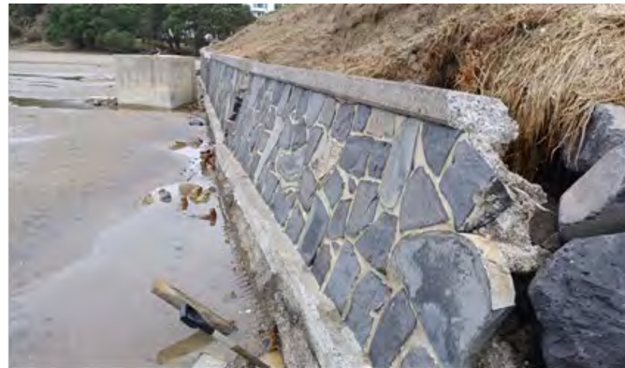
Stage 2: Failed rock masonry seawall to be replaced with a rock revetment seawall.
