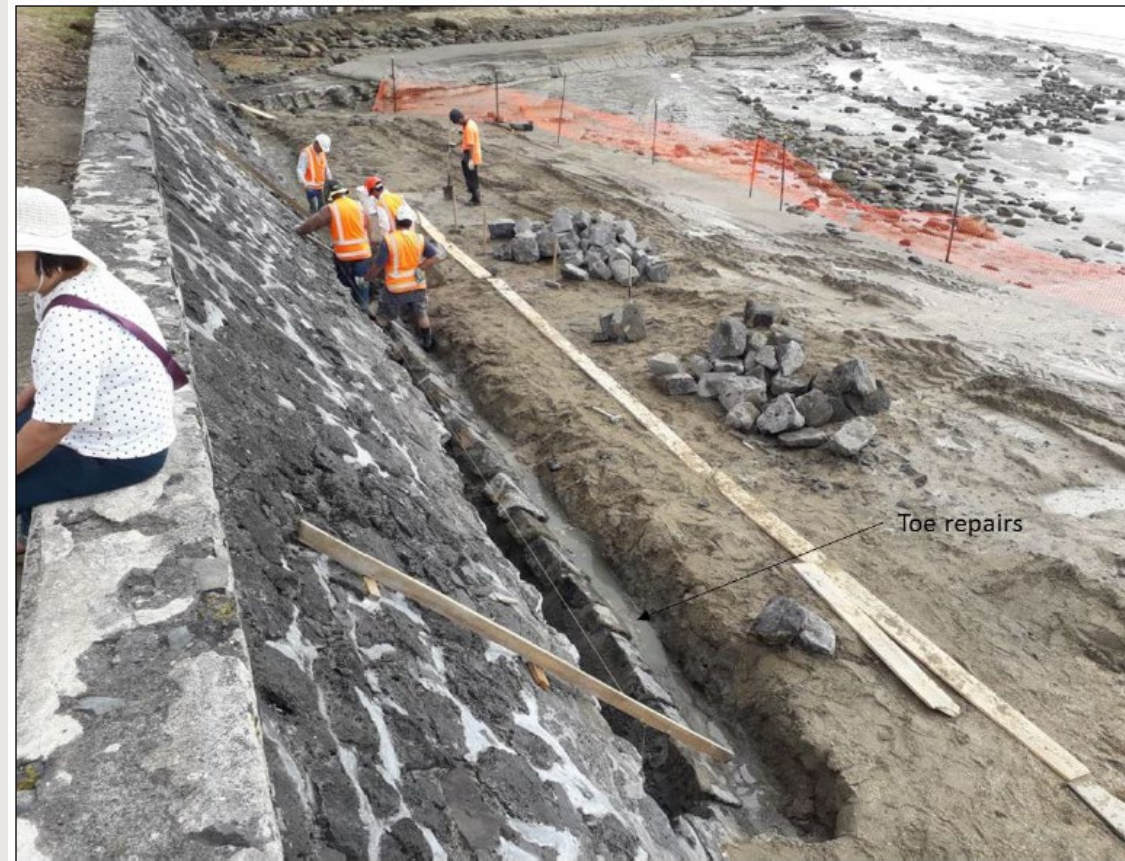
Above – seawall being repaired in recent years. Image and data supplied by Coastal Management team
