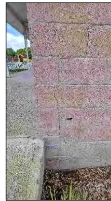
Photo 16: Northern gable end wall cracks
