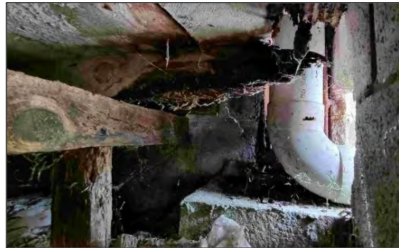
Photo 24: Rotting timber support / formwork
