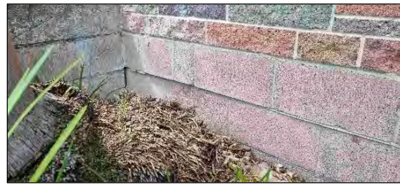
Photo 20: Foundation wall moved by Palm tree
