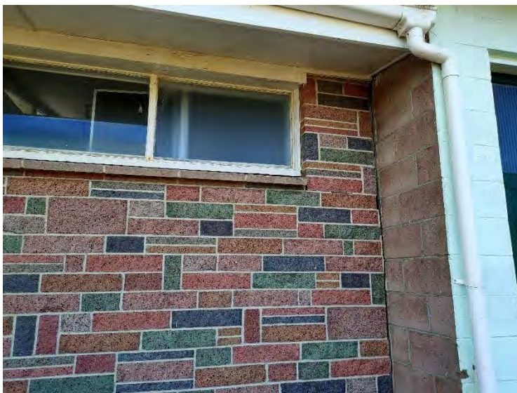
5. Large gap of the brick venner joint to the block wall
