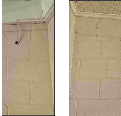
Photo 15: Playgroup return wall cracks
