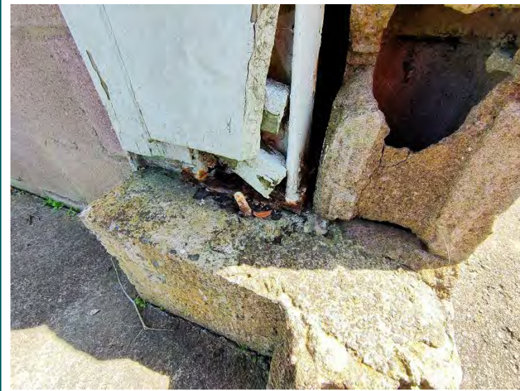
14. the broken concrete block and the UB steel column is corroded at the east-south corner (exterior)
