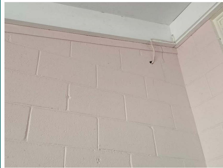
13. Crack at top of the internal concrete block wall (URM) of the play group room
