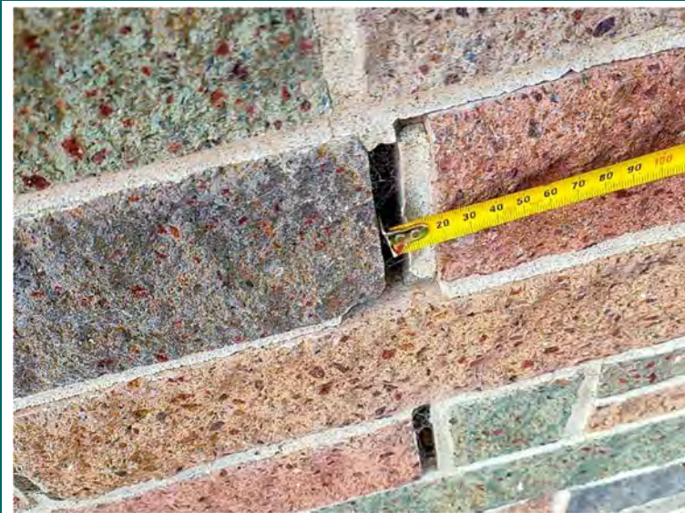
3. Crack on the brick veneer (The foyer & toilet block)
