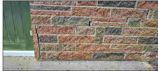
Photo 18: Brick veneer stepped cracks
