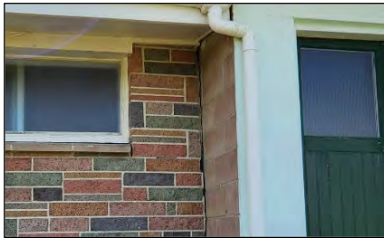
Photo 19: Gap at western return wall
