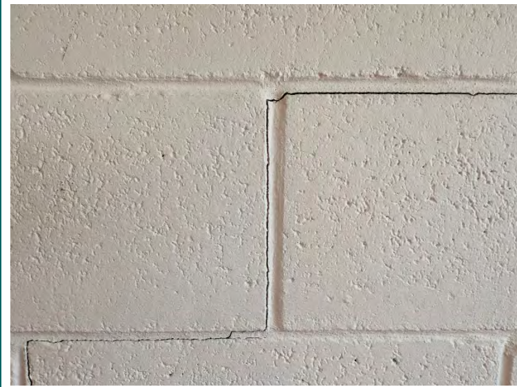
12. Crack on the URM gable wall
