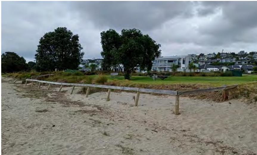
Image to left : Storm damaged barrier
