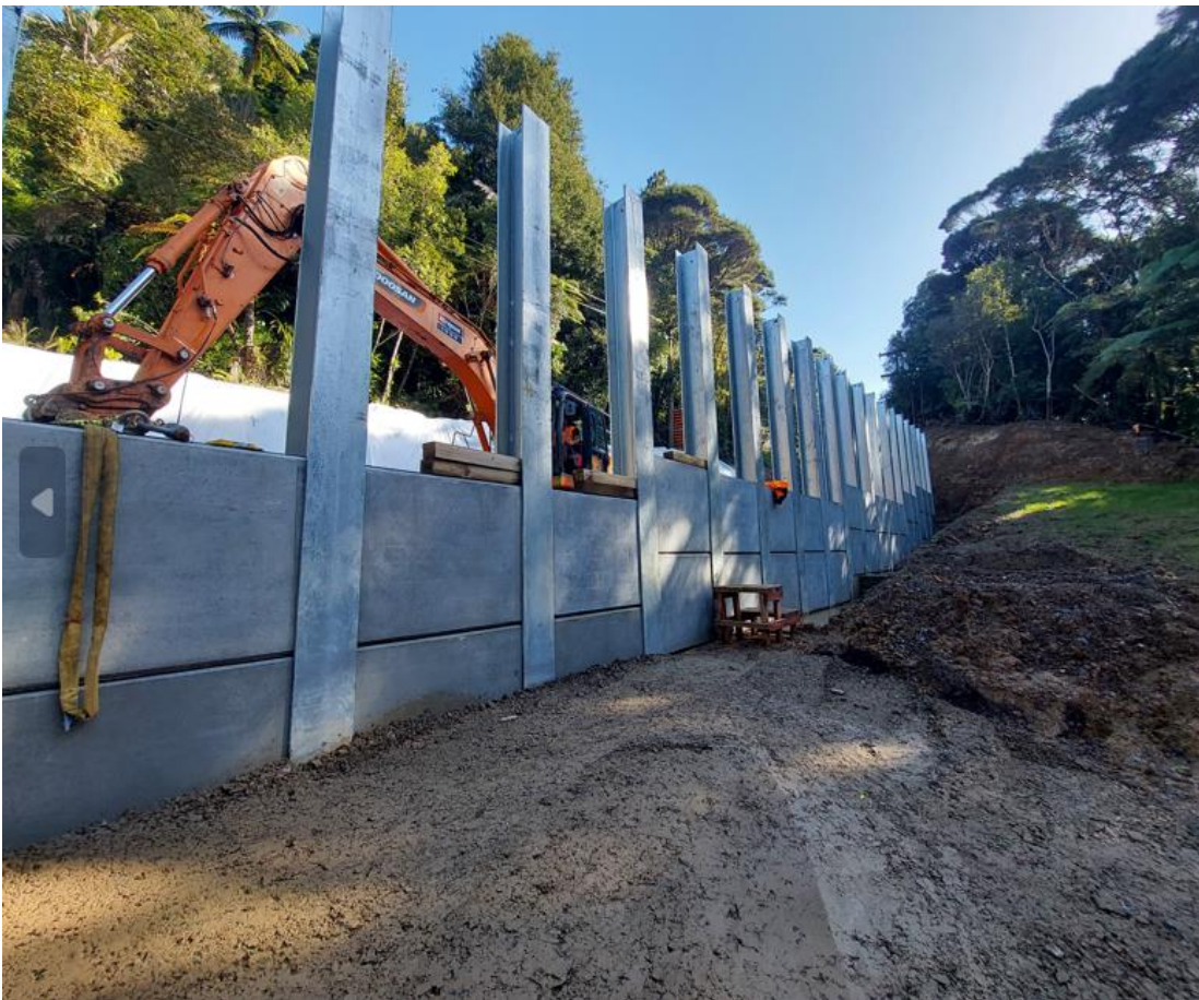
Retaining wall construction on the site on Scenic Drive, just past Arataki
