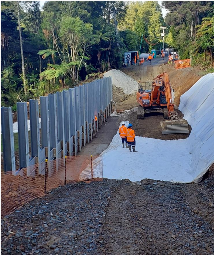
Works progressing, once culvert works are completed the final three piles for the retaining wall will be installed at the far end of this site.
