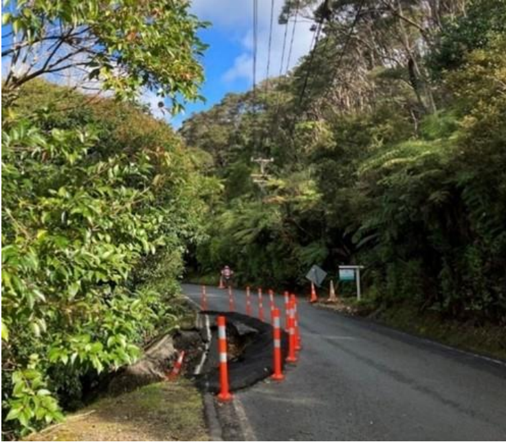
Under slip at Kellys Road
