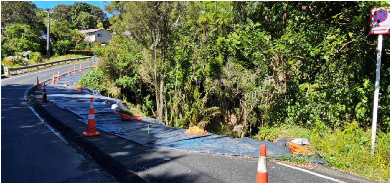
Woodlands Park Road slip site
