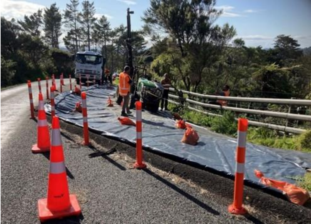
Wairere Road slip site
