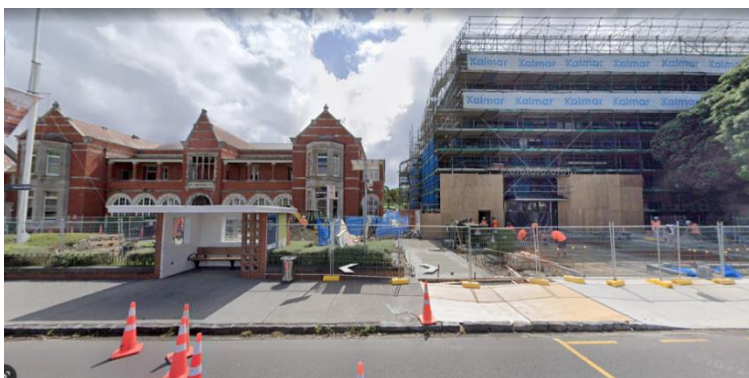
Figure 21 Construction of The foundation Parnell near to Jubilee building currently functioning as a Parnell Library.
