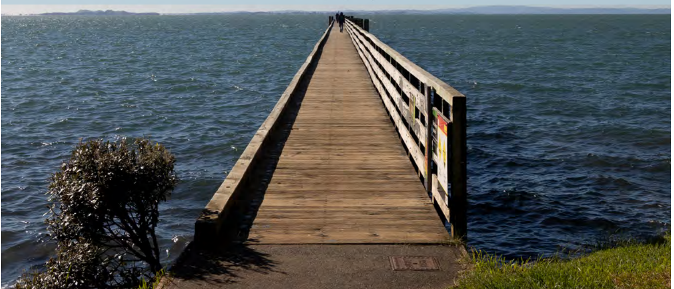
Image: Cornwallis Wharf, Cornwallis (Category B ID 00148). Built 1900. © Rachel Ford (Heritage Unit, Auckland Council, 2024)
