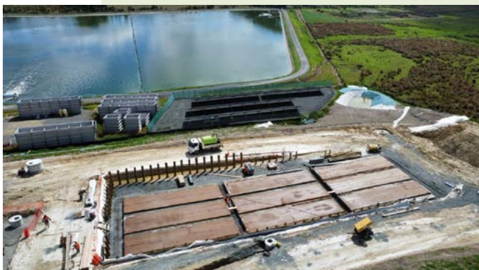
▲ Wellsford water treatment plant
