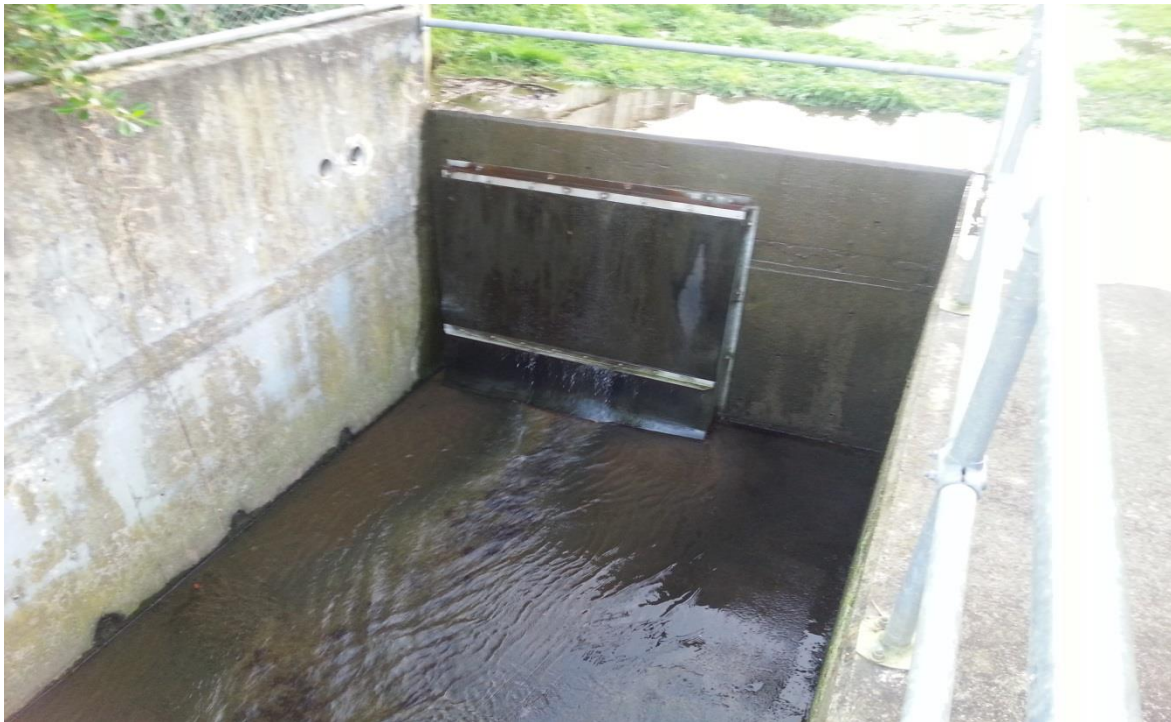
Figure 3-1 Flap Gate at the 1600mm Diameter Culvert Outlet at Haverstock Road Reserve
