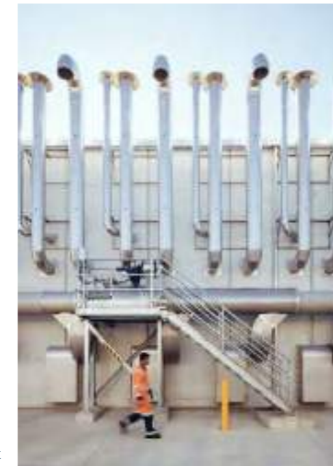
► Māngere Wastewater Treatment Plant
