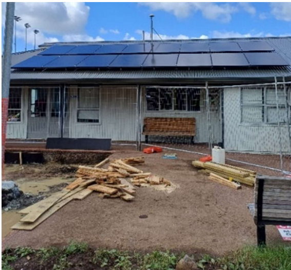
Figure 4 Glendowie Community Centre now uses Solar Photovoltaic Cells providing low-cost energy while reducing carbon
