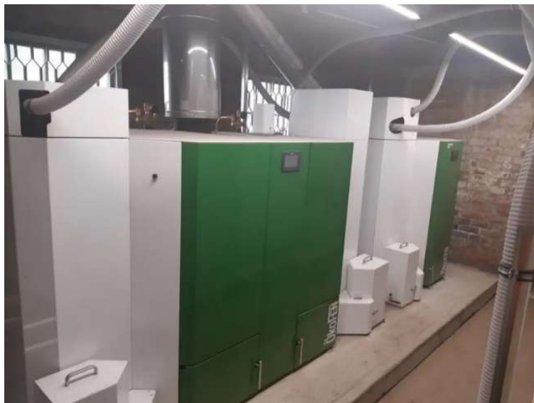
Figure 6 ÖkoFEN PES 128 and PES 64 Pellet Boiler Cascade System
