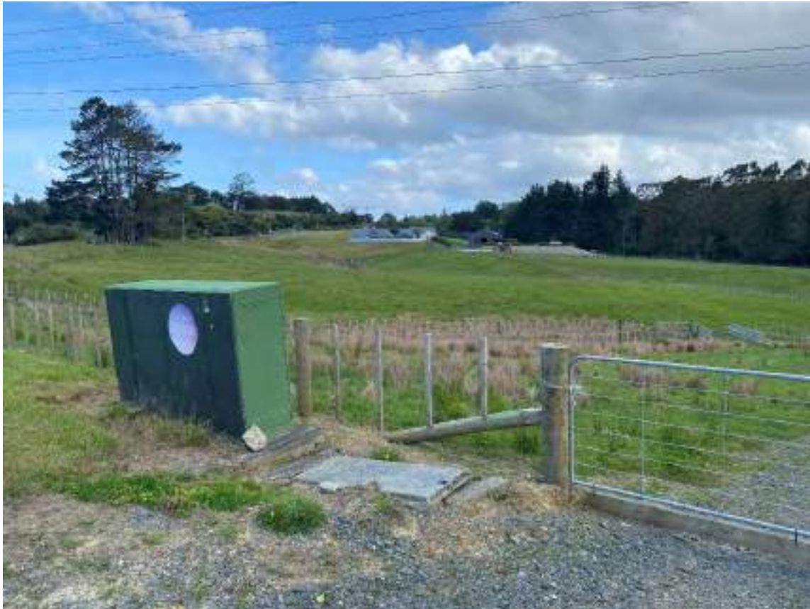
Figure 6: Site looking south-east of 836 Sandspit Road – transformer was not audible during noise measurement
