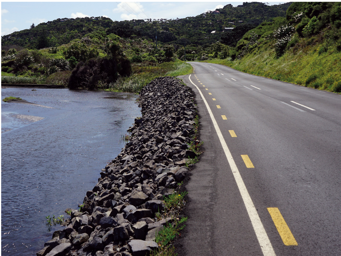
Integrated infrastructure response near Bethells beach.
