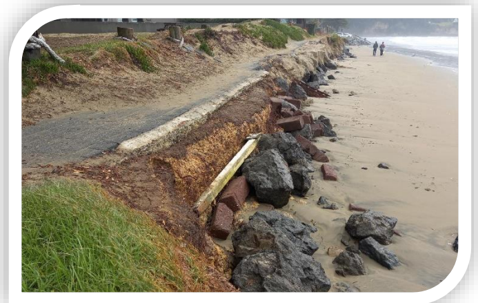
The existing walkway after a storm event
