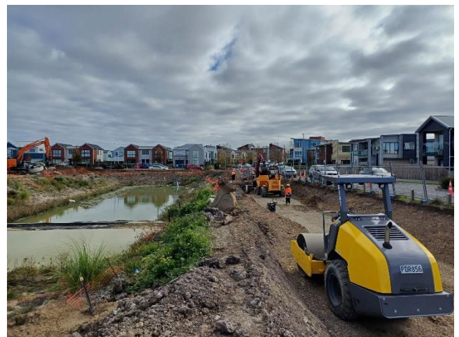
Photo: Installation of stormwater pipes and manholes along the Squadron Drive boundary, June 2024
