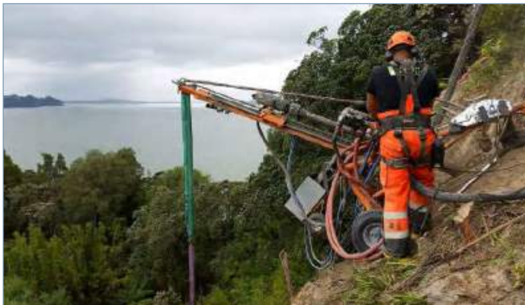
Figure C-5 Example of typical small, roped access rig used to install anchors or nails on steep slopes.
