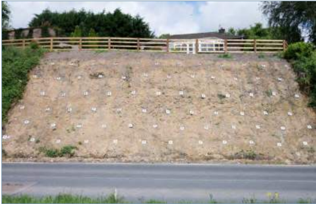
Figure C-6 Example of surface erosion prevention matting and mesh for use with soil nails on relatively steep slopes.
