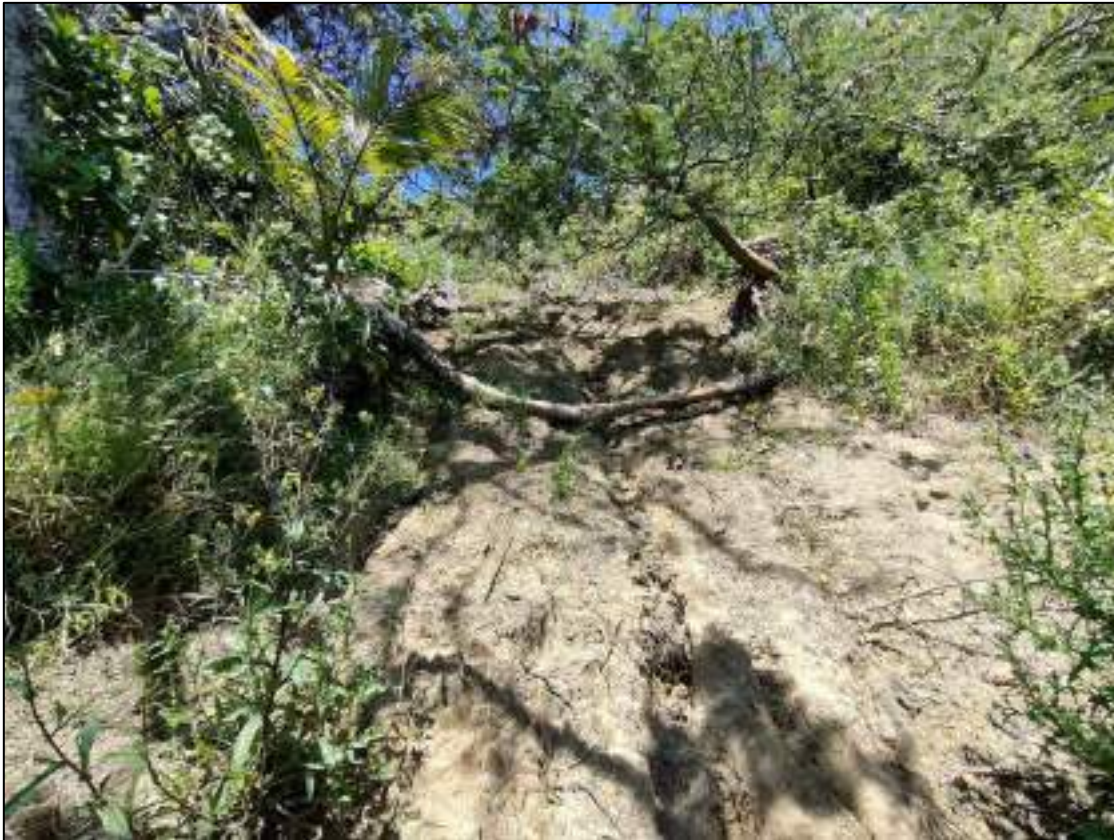
Figure 2.9 Failure surface (evacuated zone) exhibiting evidence of post failure erosion. Looking upslope.
