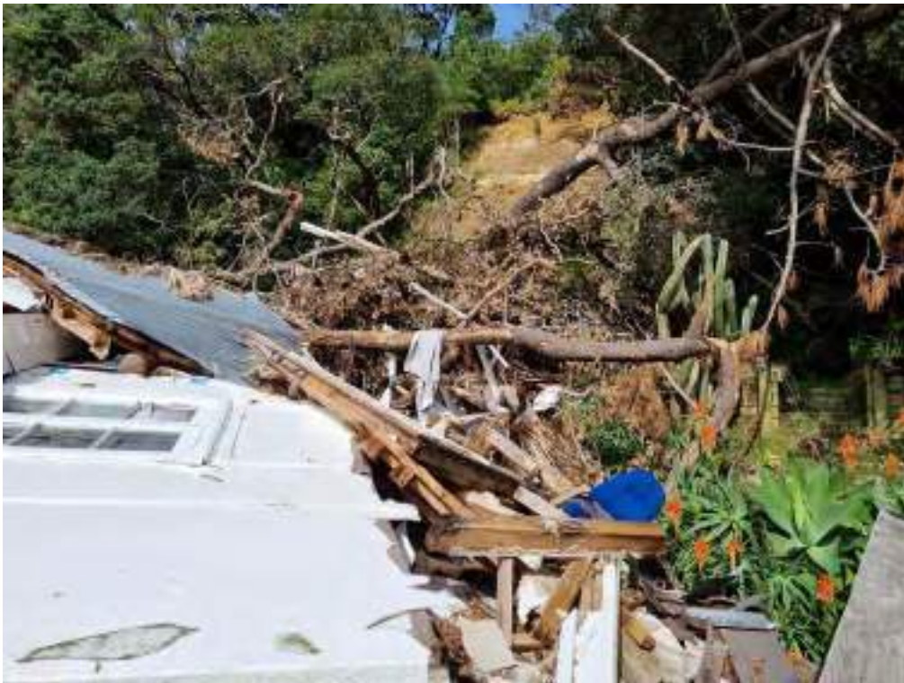
Figure E4 Example of a dwelling on Domain Crescent completely destroyed by landslide with large pile of accumulated vegetation debris on upslope side.
