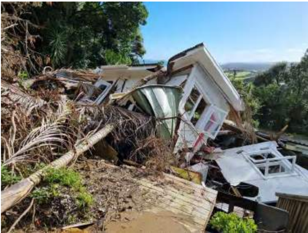
Figure E5 View of upslope side of completely destroyed timber frame dwelling. Note large pile of accumulated vegetation debris on left.
