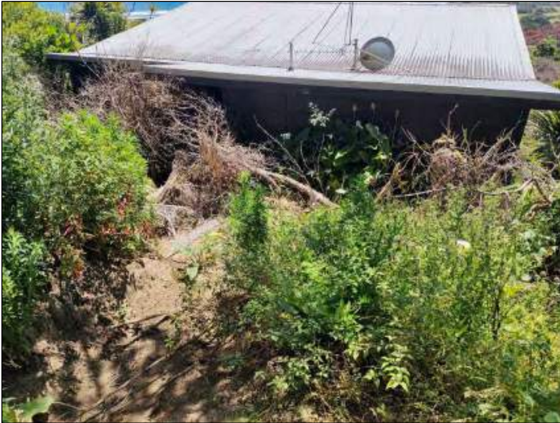
Figure 2.10 Debris piled up at the rear of dwelling (estimated up to 1.5 m thick)
