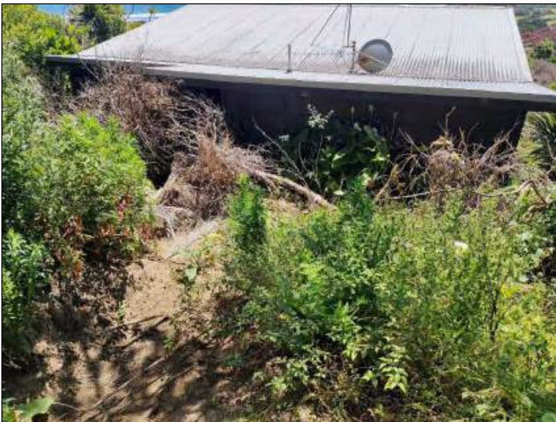
Figure 2.10 Debris piled up at the rear of the dwelling at No. 85 Domain Crescent (estimated up to 1.5 m thick)
