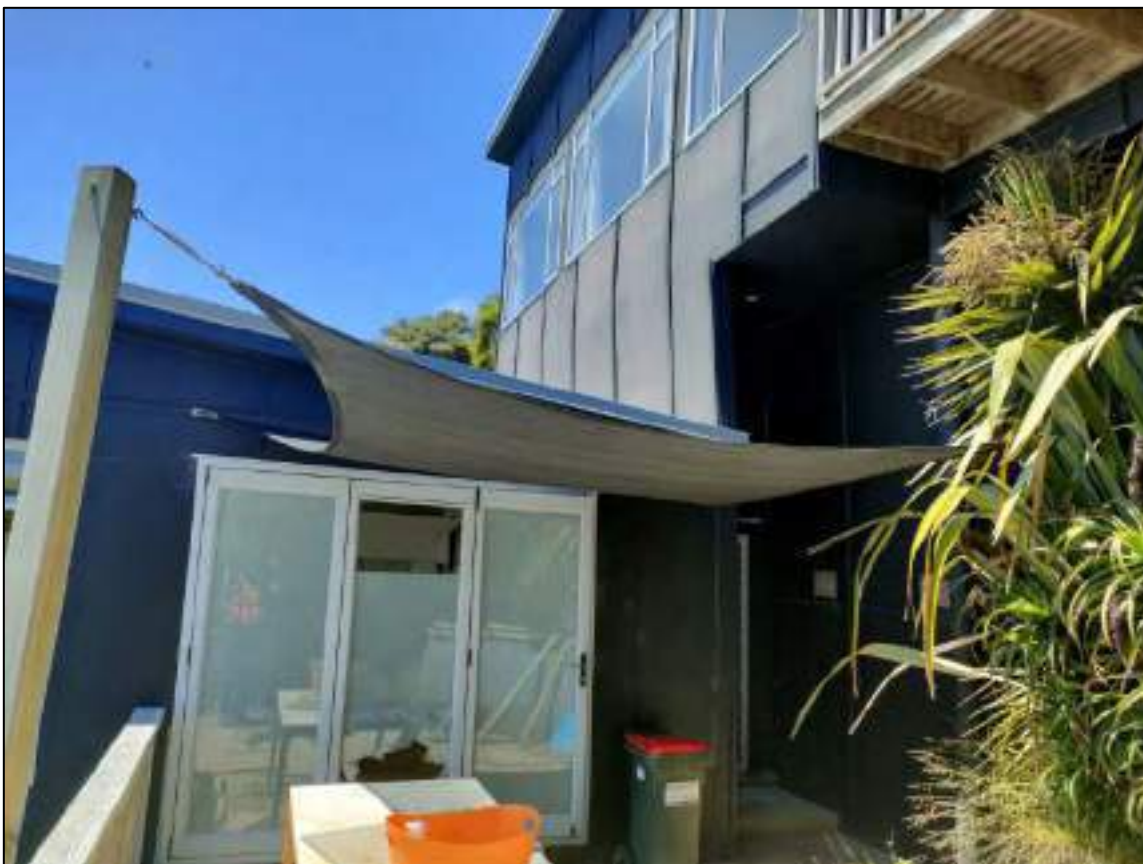
Figure 2.11 Damage caused by landslide includes racking of entire building (exhibited by bending of exterior wall)
