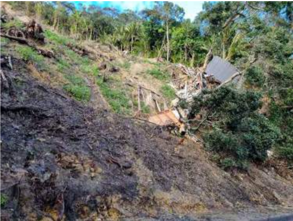
Figure E7 View of remains of completely destroyed house on slope above Motutara Road. Note mixture of soil debris and vegetation.
