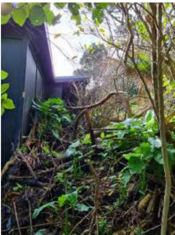
Figure E13 View of upslope side of dwelling pictured in Figure E12 showing accumulated landslide debris against rear wall.
