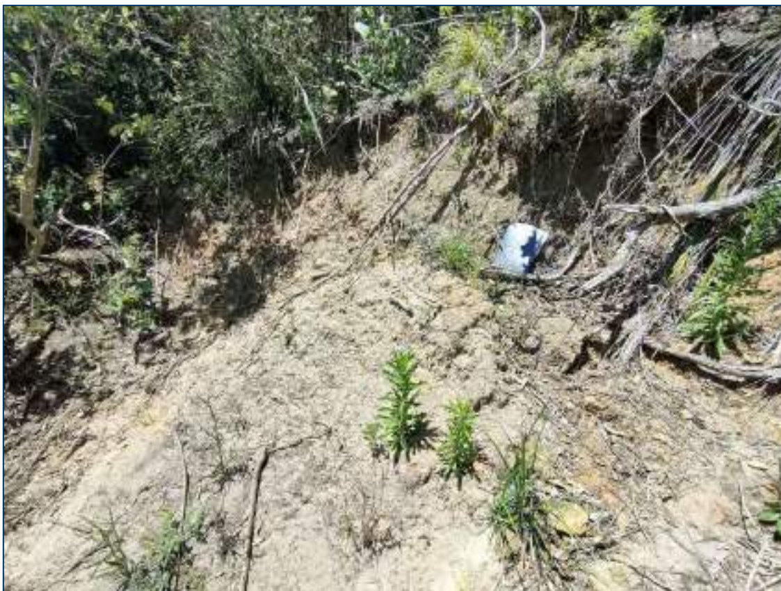
Figure 2.8 Exposed headscarp of landslide.
