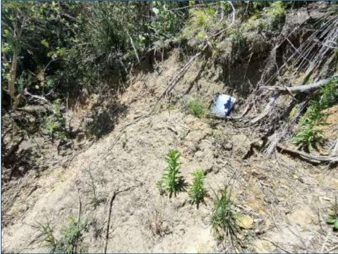
Figure 2.8 Exposed headscarp of landslide.
