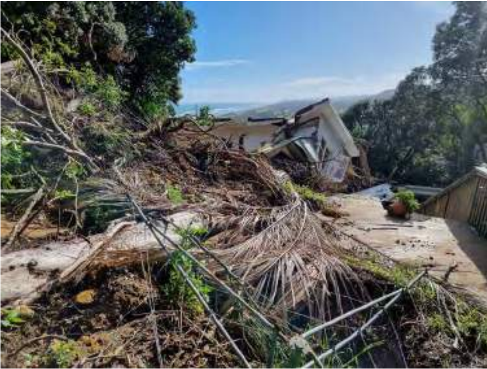
Figure E6 View of the same dwelling pictured in Figure E5 taken further upslope. Note mixture of soil debris and vegetation. Residence has been moved several metres downslope.
