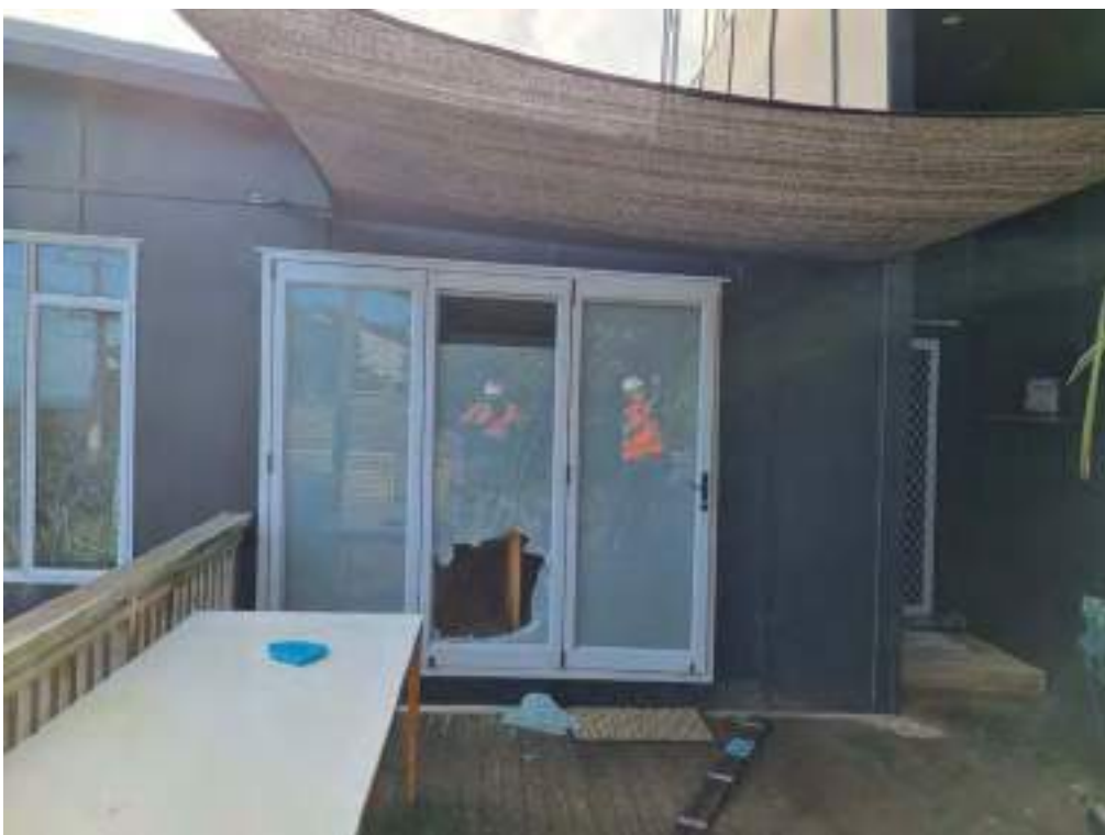
Figure E12 Side view of home above Motutara Road. Note tilting of upper storey wall and deformed window frame.
