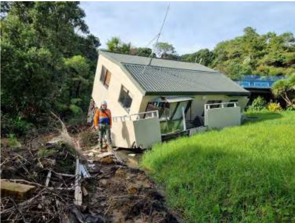
Figure E9 Example of a dwelling on Domain Crescent where ground floor of the structure has collapsed causing house to topple over with the upper storey remaining largely intact.
