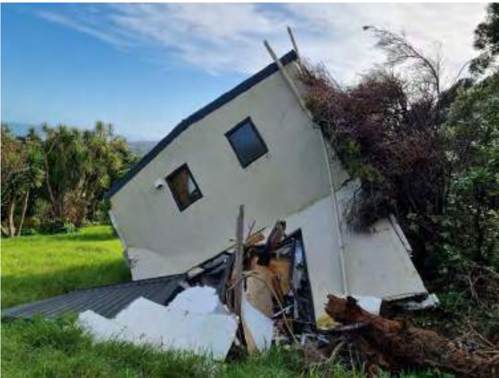
Figure E10 View of side profile of dwelling pictured in Figure E9, showing collapse of the ground floor and build-up of vegetation debris at rear.
