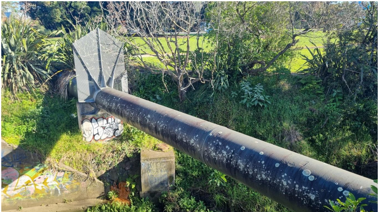
Figure 18. View looking west over pipe crossing on the northern side of the Walmsley Road bridge
