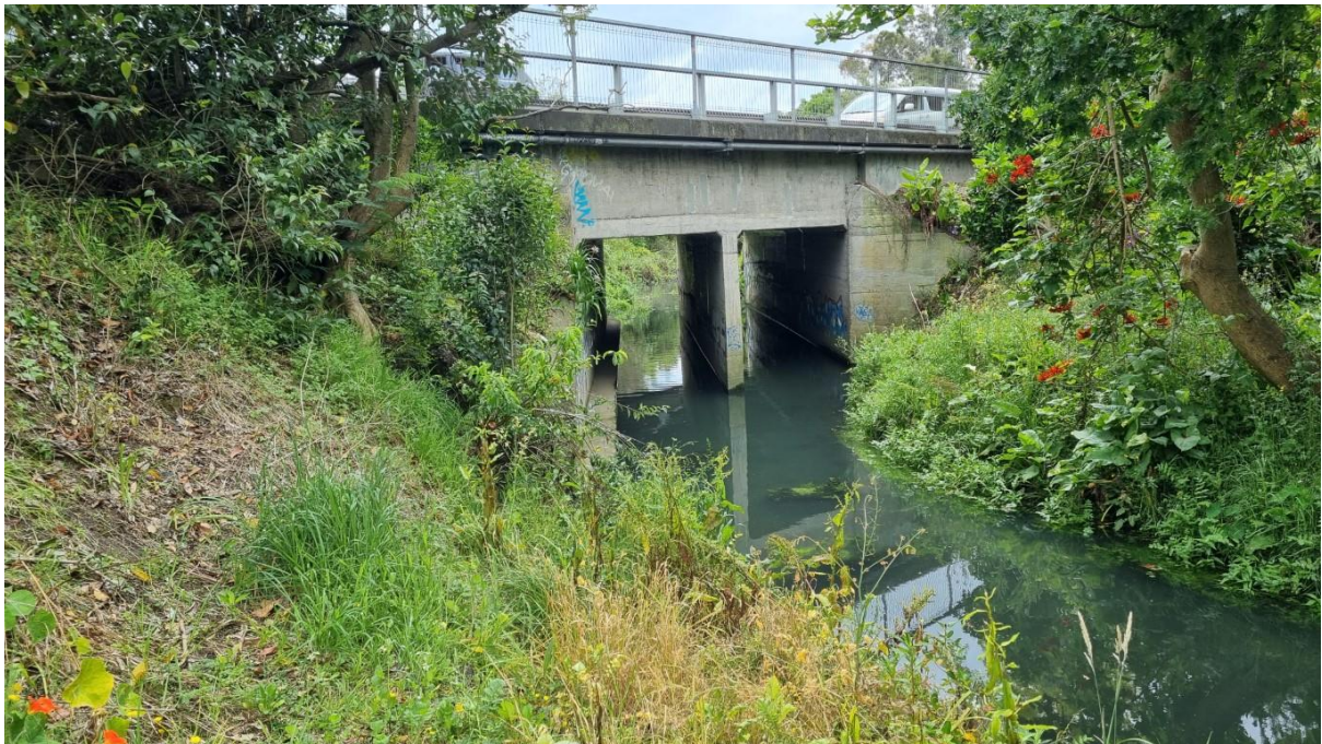
Figure 16. View looking north towards the southern side of the existing Walmsley Road bridge
